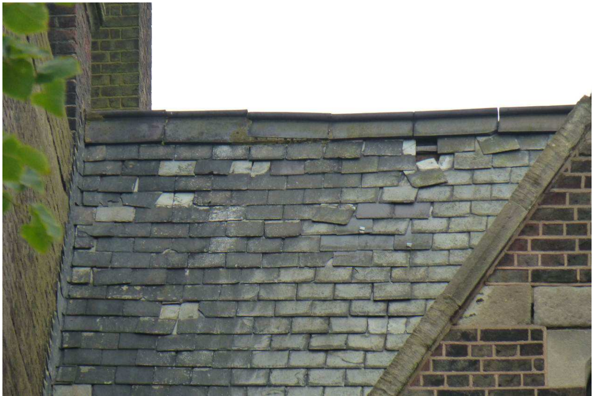
Photo 11. Main roof, north elevation areas of slipped slates.
