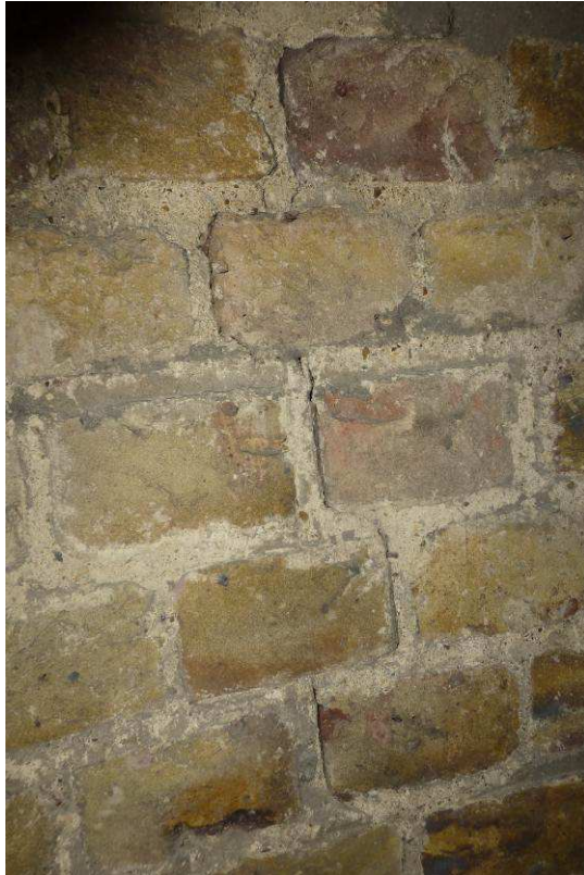
Photo 6. Vertical cracking to tower staircase
