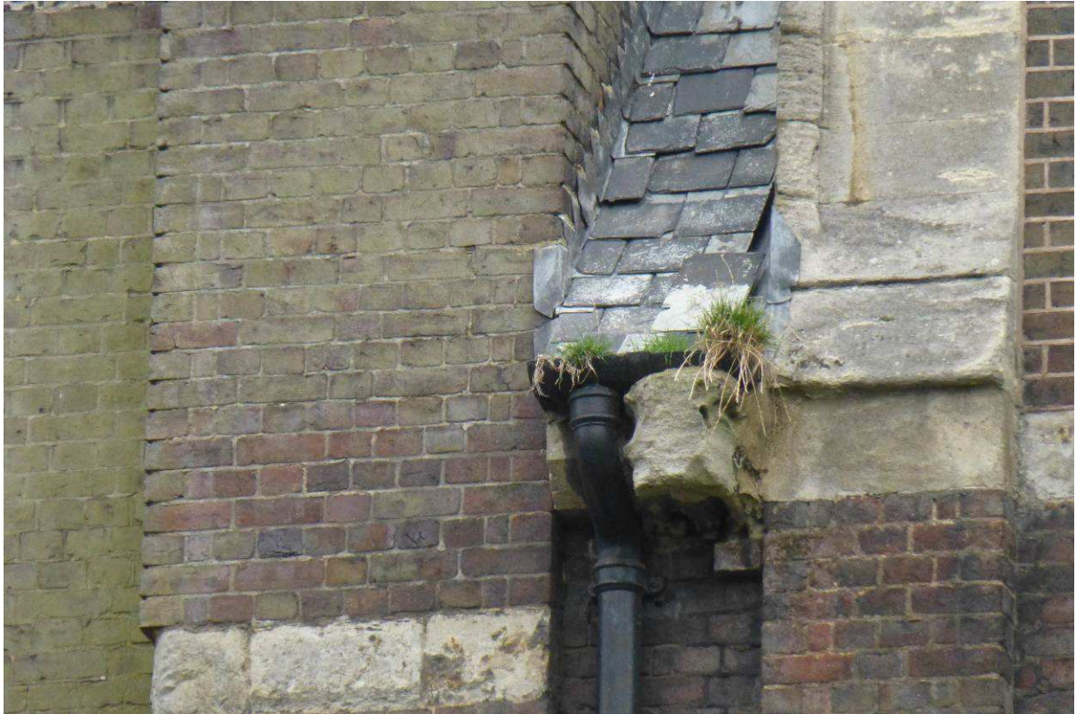
Photo 8. Vegetation and slipped tiles on north elevation adjacent to tower.
