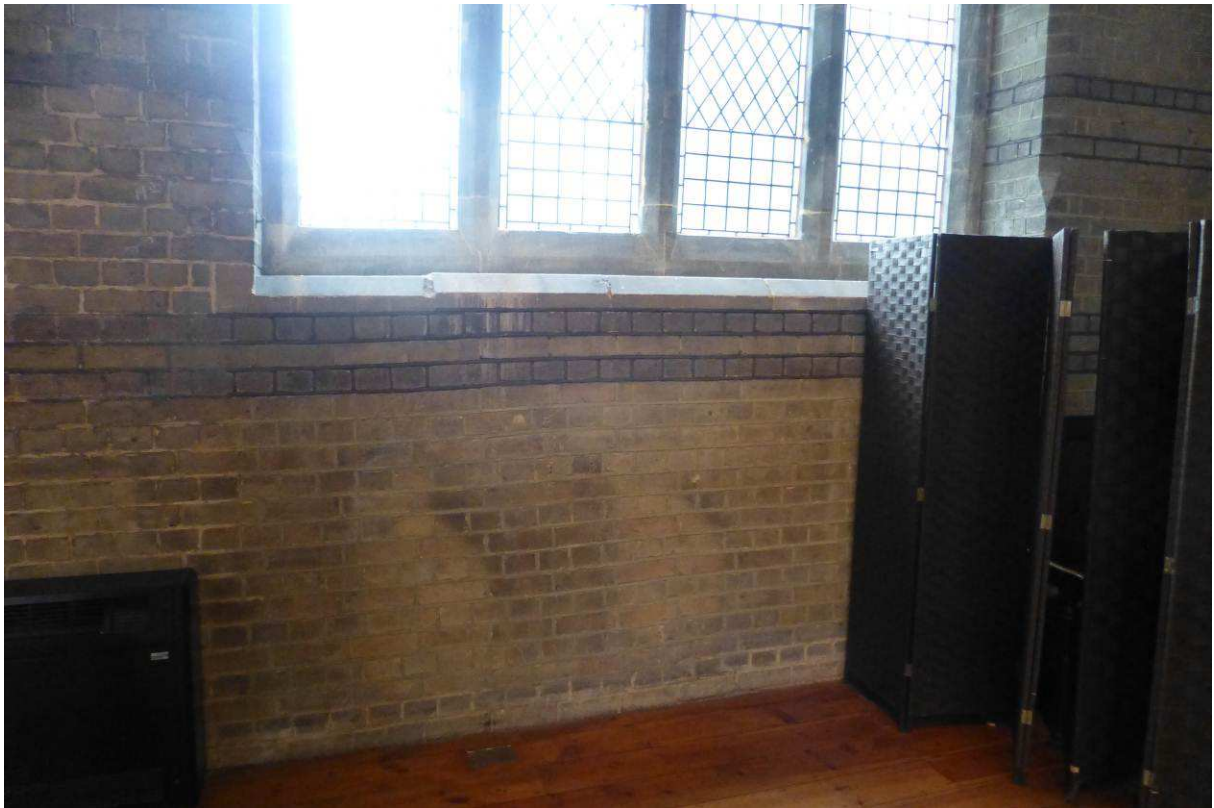
Photo 3. Distortion to the east end of the north aisle internally
