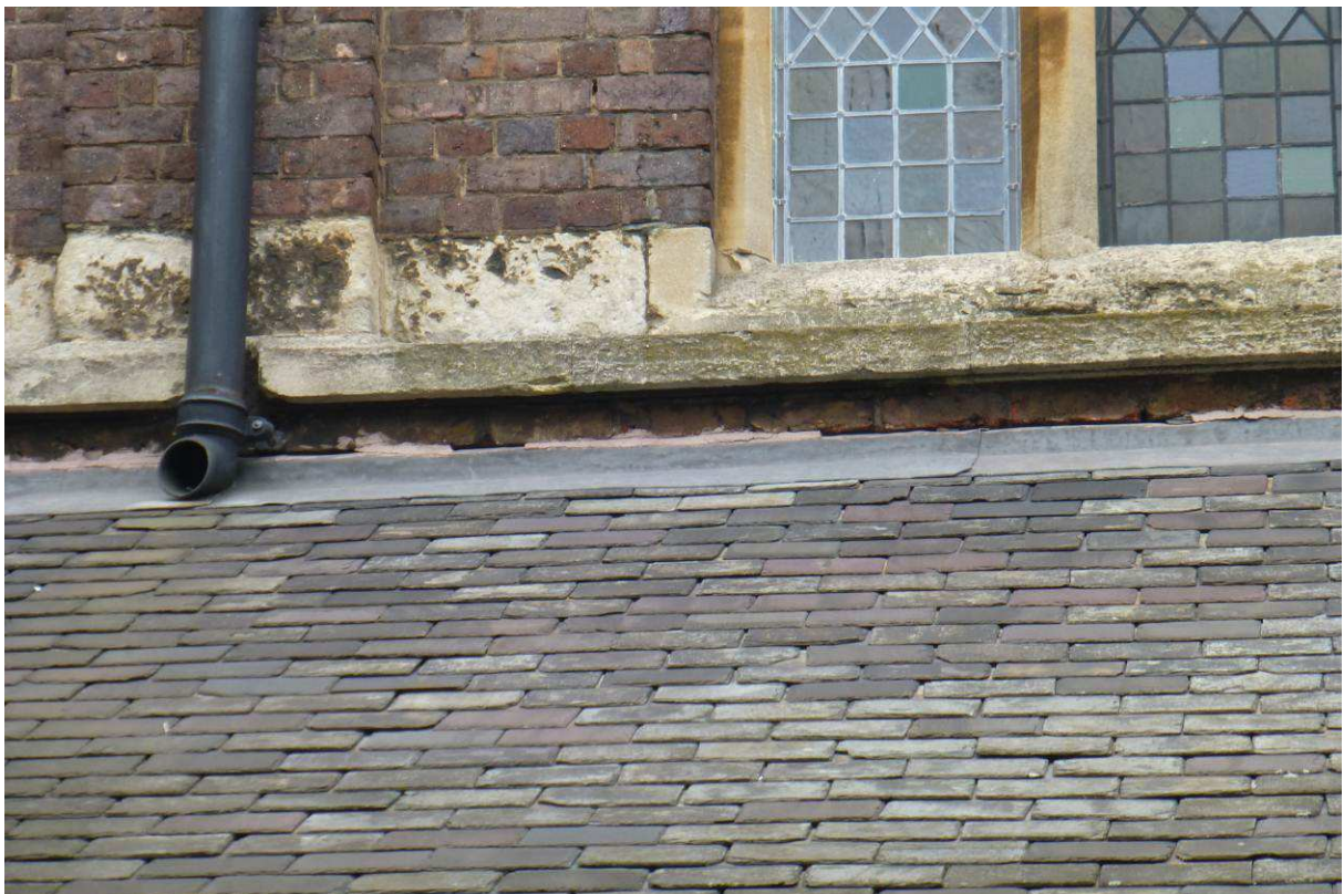
Photo 9. Failure of mortar fillet between south aisle roof and clerestory wall.
