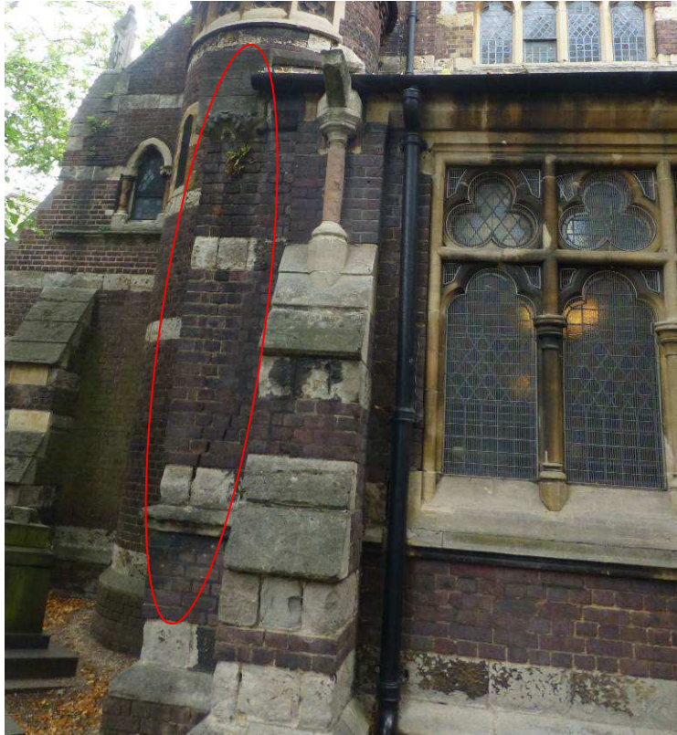
Photo 4. Cracking and vegetation to south porch
