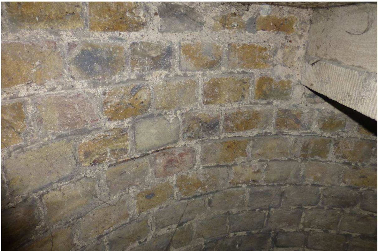
Photo 7. Horizontal cracking in the tower staircase
