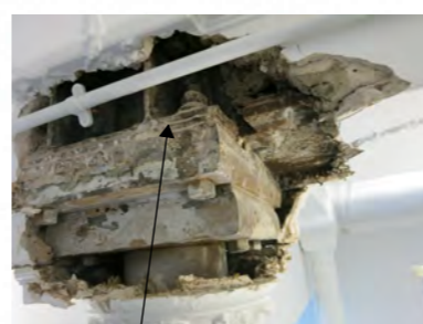
60mm capping plate to 200 diameter circular column with 420x370 capping plate. Beam 350 wide.
