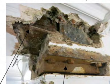
360 wide beam formed with double web x 370 deep Column head 370x410 on plan, formed from 70mm plate. 200 diameter circular column under
