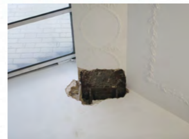
230 square column observed supporting 350w beam. Column transfers again at mid height to avoid window opening.
