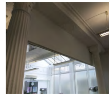
Architecturally encased column and beam. Tbc if investigations can locally remove cornice detail.
