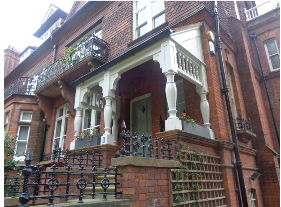
Figure 17: Reinstated timber porch – spindles to the side. Ironwork has all been refurbished.
