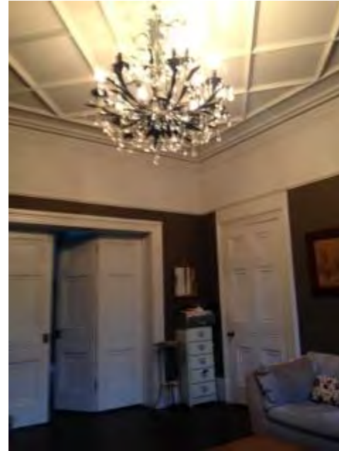
Figure 24: Stapwork plaster ceiling, cornices and picture rail in the front room at ground floor level.
