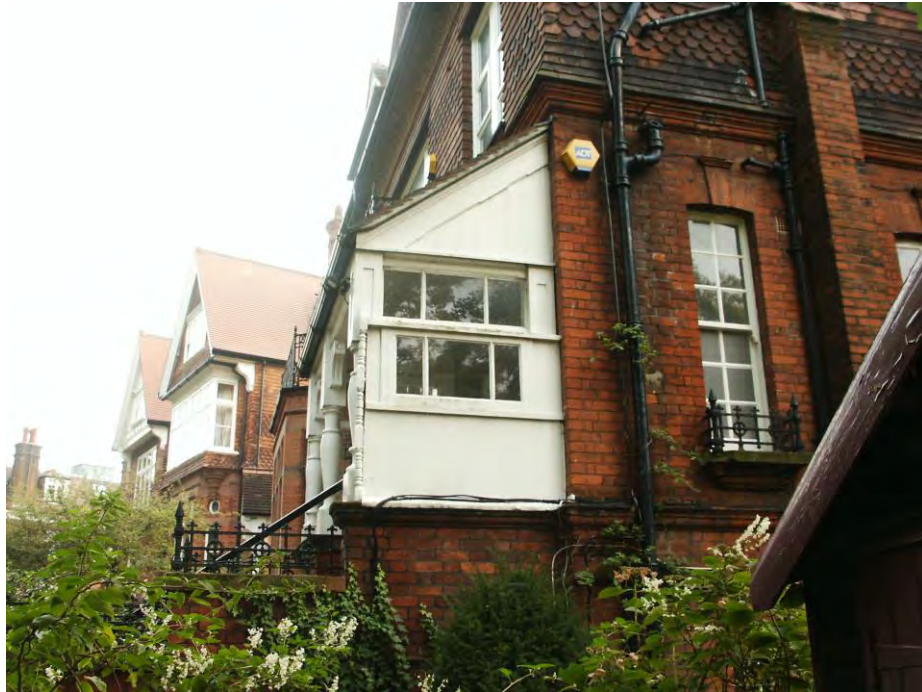
Figure 16: Photograph taken prior to restoration works. In the foreground the opening to the side of the porch is visible. It is clear the original spindles had been removed.
