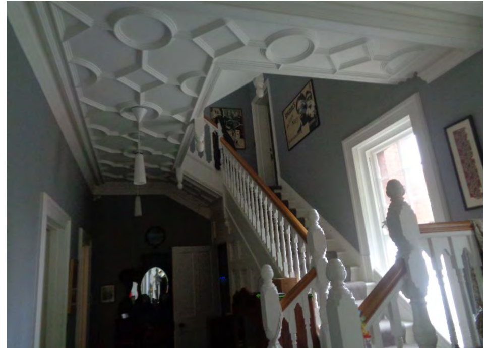
Figure 14: Reinstated strapwork plaster ceiling and fully restored/replaced lower flight in entrance hall
