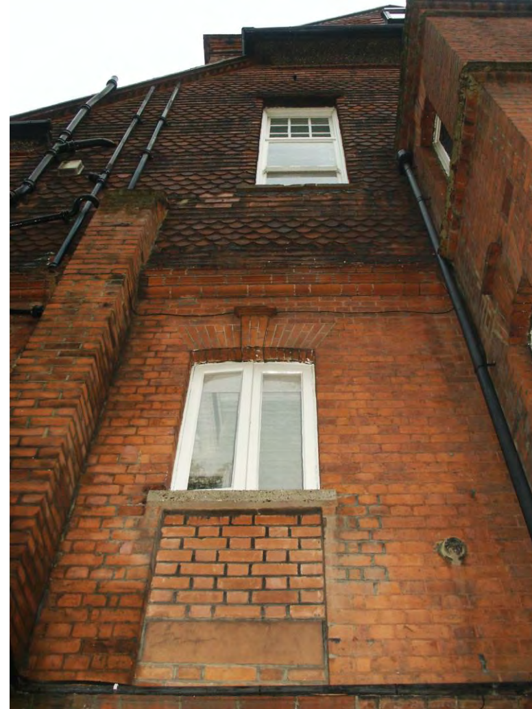
Figure 19: UPVC window and blocked opening before new opening was installed. Redundant pipes were also removed.
