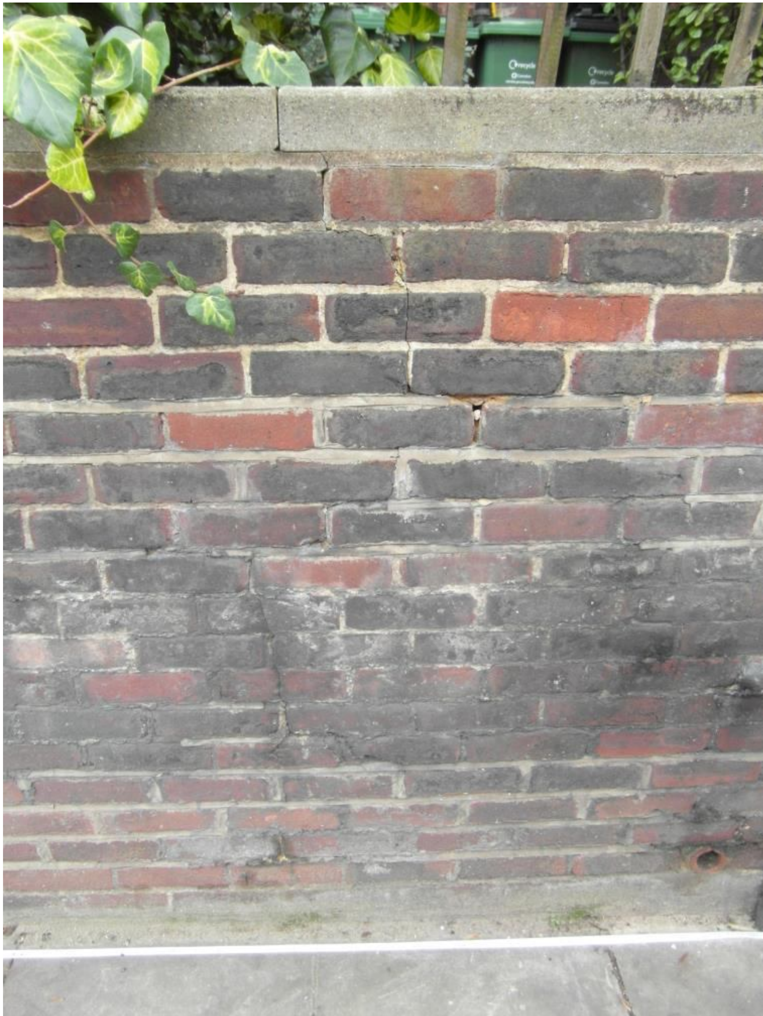
Cracks at 5 metres
