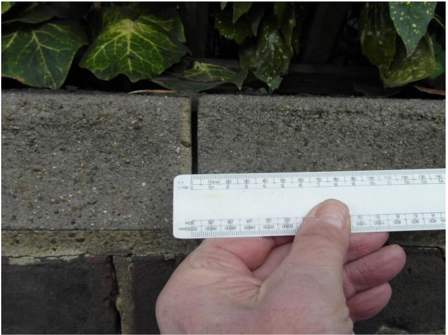
Cracks at 2 metres
