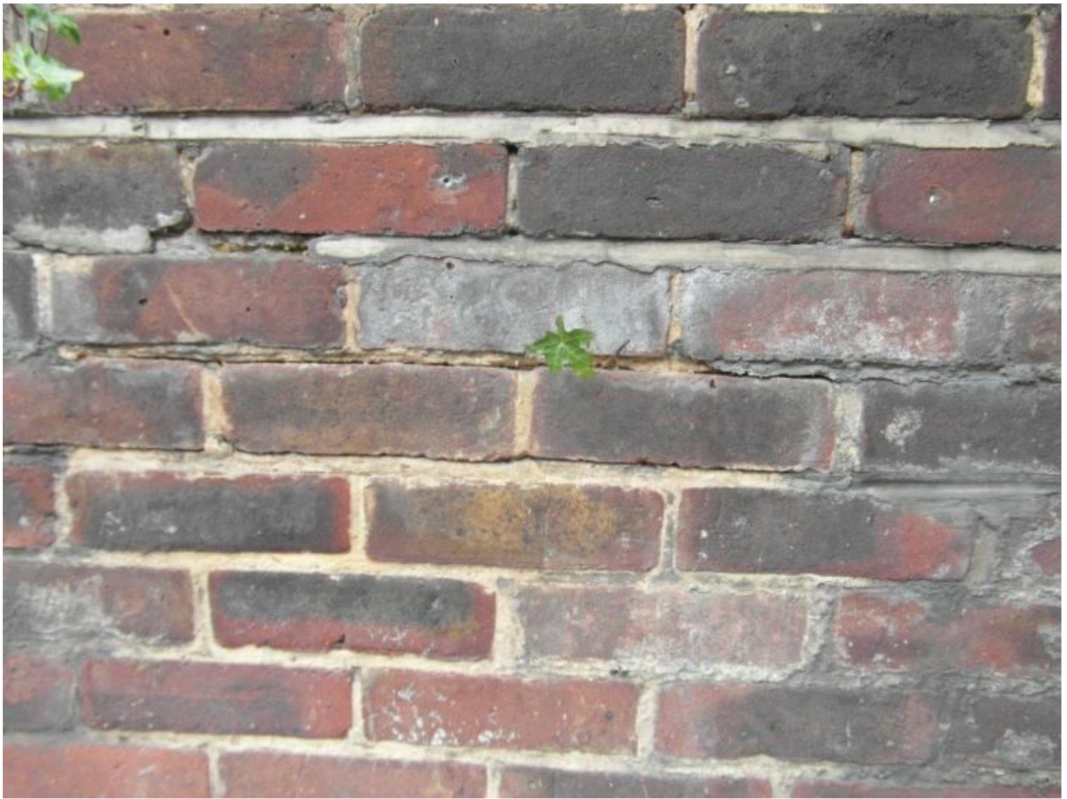
Finchley Road Retaining Wall Horizontal cracks at 10 metres
