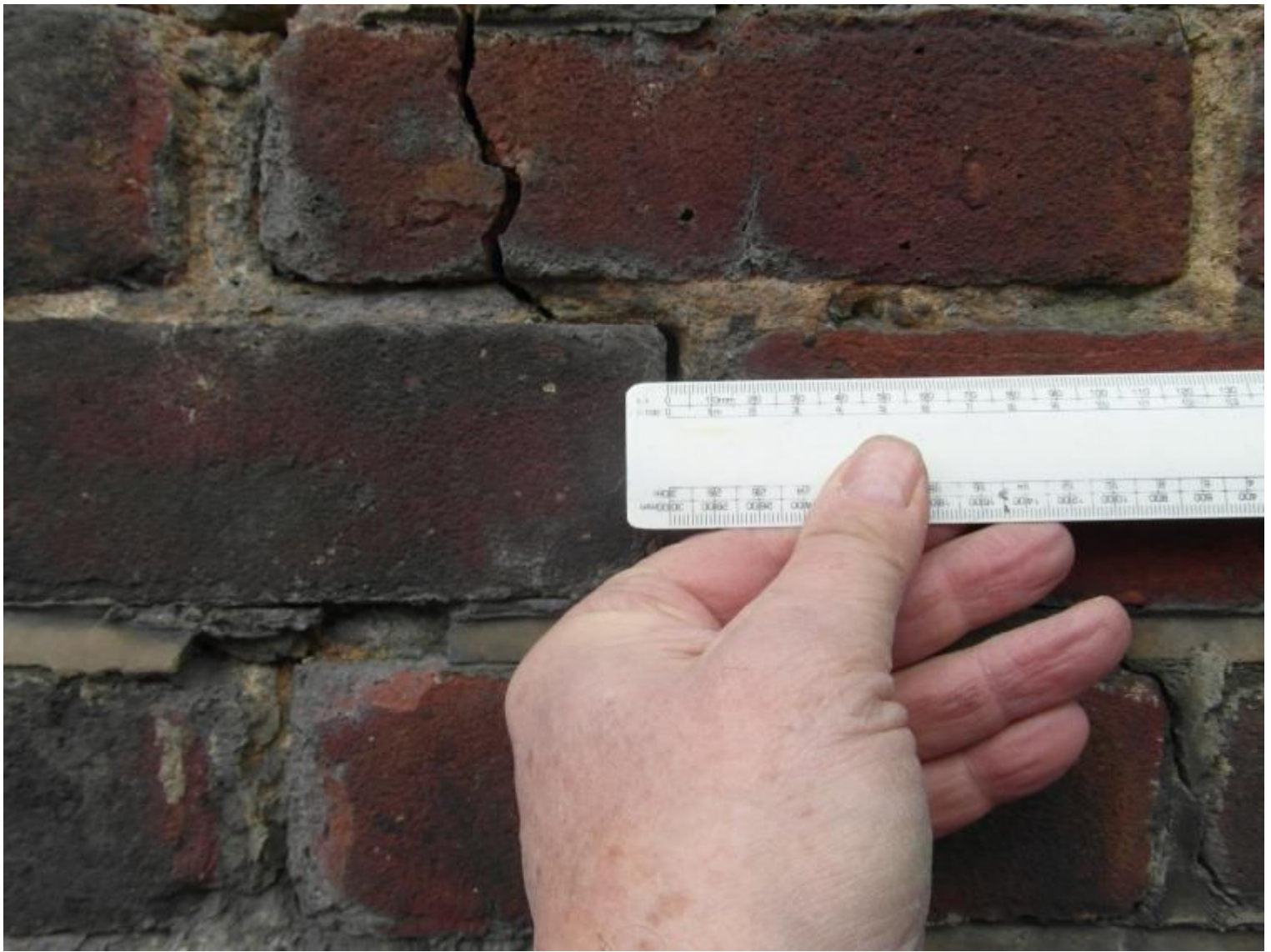
Cracks at 9 metres
