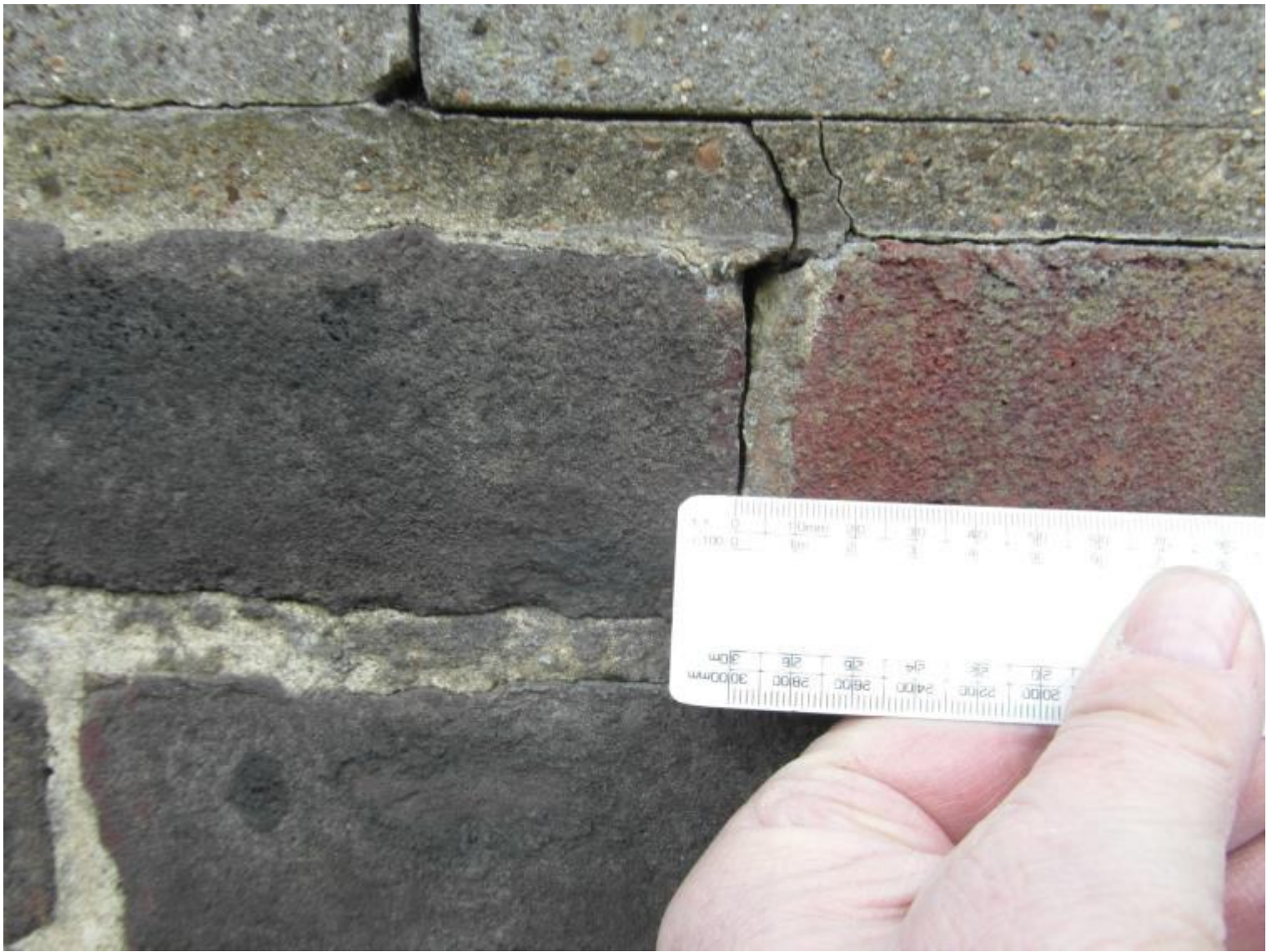
Cracks at 5 metres
