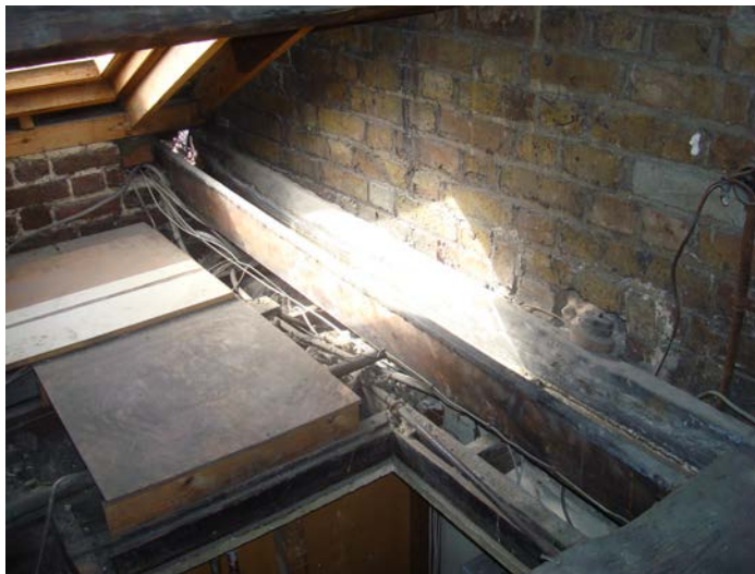
fig.11a Ingress of lead gutter along the now party wall
