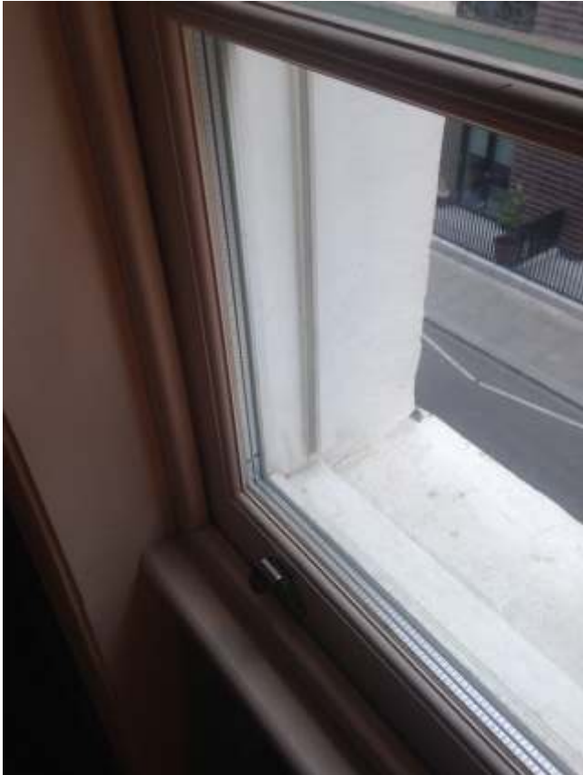
Appendix 1.7: View of bottom rail and furniture to new timber sash window.
