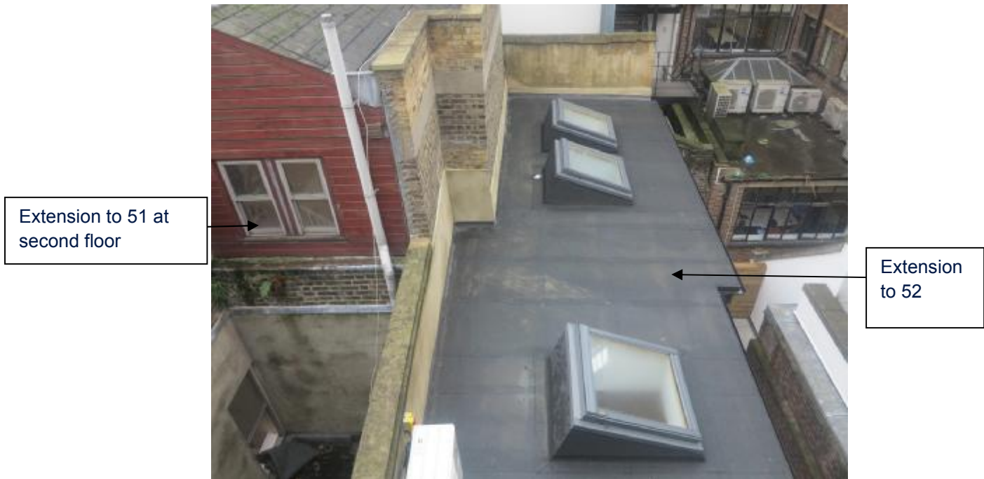
Image above: View of extensions to the rear of 52 Tottenham Court Road
