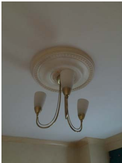
4 | THIRD FLOOR FRONT LEFT BEDROOM CEILING ROSE
