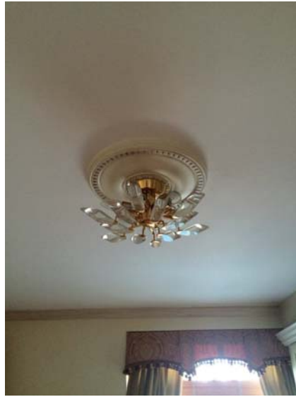
5 | THIRD FLOOR FRONT RIGHT BEDROOM CEILING ROSE
