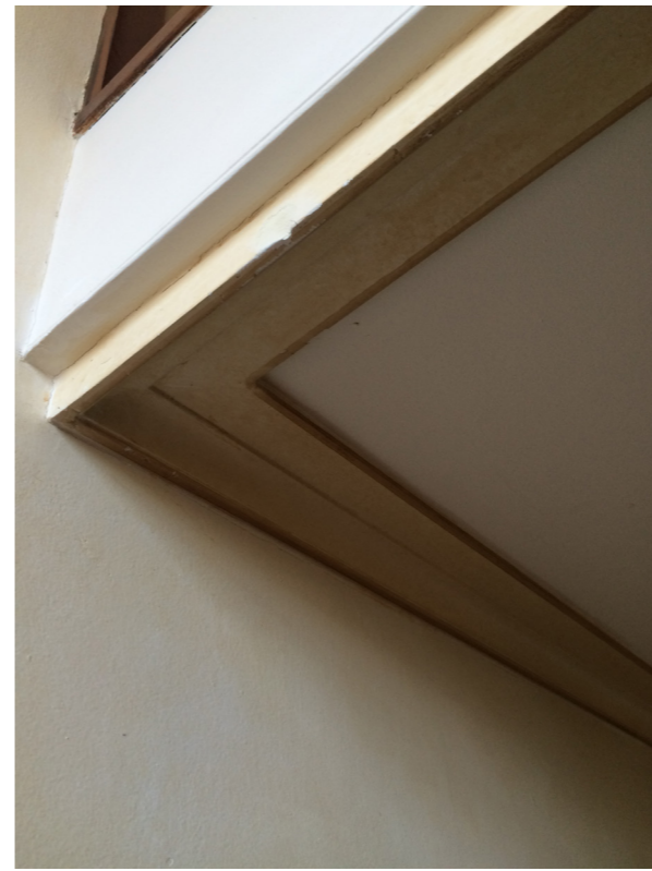
3 | FIRST FLOOR STAIRWELL COVING
