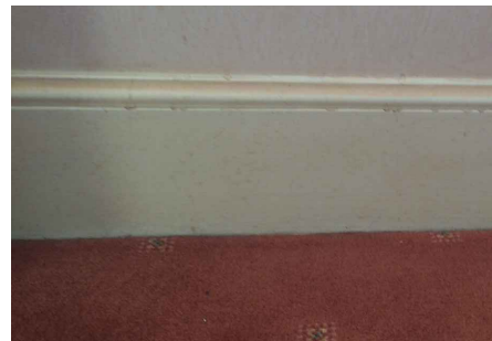
07 EXISTING SKIRTING IMAGE THIRD FLOOR EXISTING THIRD FLOOR LANDING (TYPICAL THIRD FLOOR)
