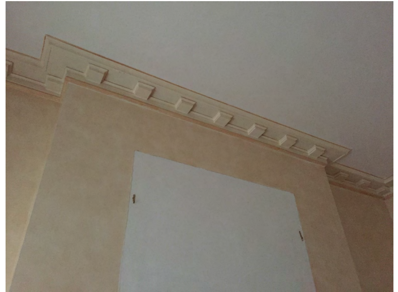
Plate 5: Ground Floor front room cornice to be replicated
