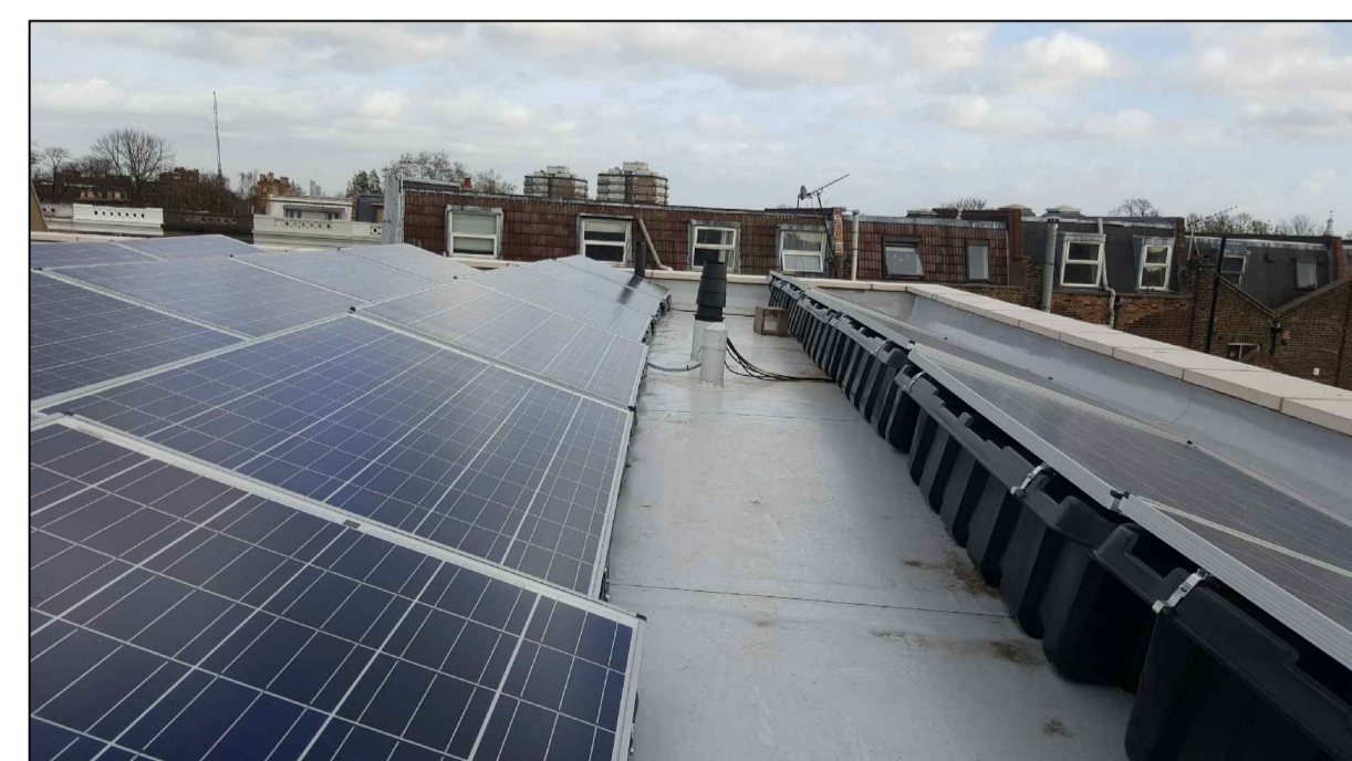
PHOTO OF AS-INSTALLED 6.5KW (26 PANELS) PHOTOVOLTAIC CELLS ON FLAT ROOF
