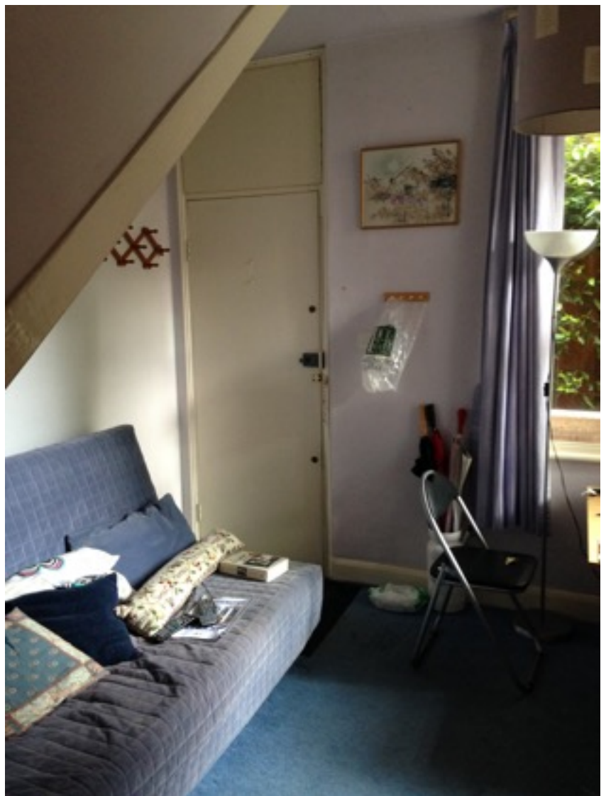
Existing external door to living room of smaller flat to be replaced
