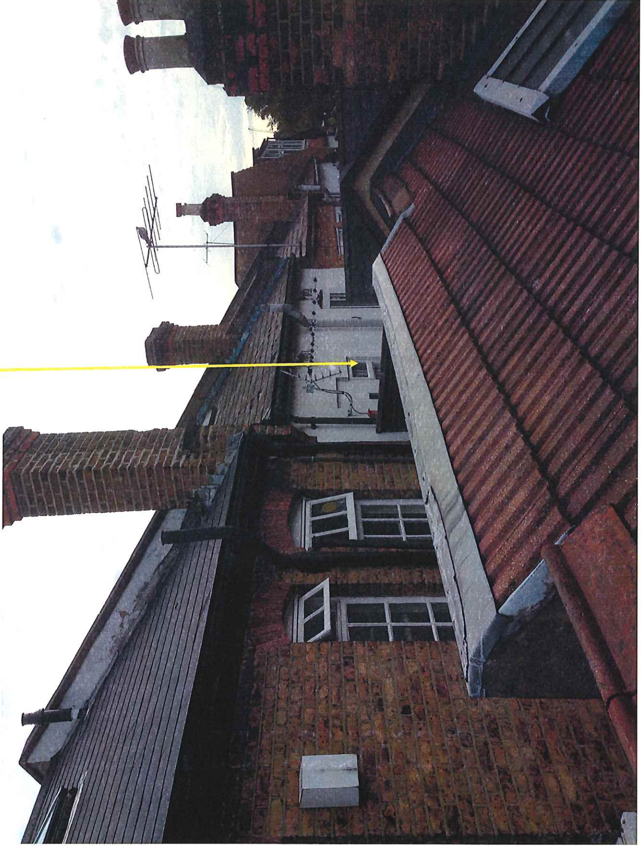
Photo B: View "B" on drawing No.M03(P1) showing windows at rear of neighbouring flats
