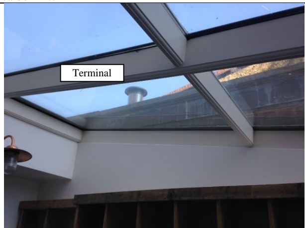
C - Terminal vent above AC outhouse
