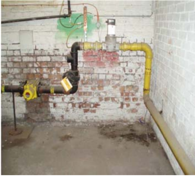
Image 9: Staining in Boiler Room
