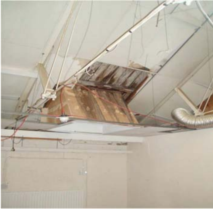
Image 13: Roof in Poor State of Repair (Disused Building)
