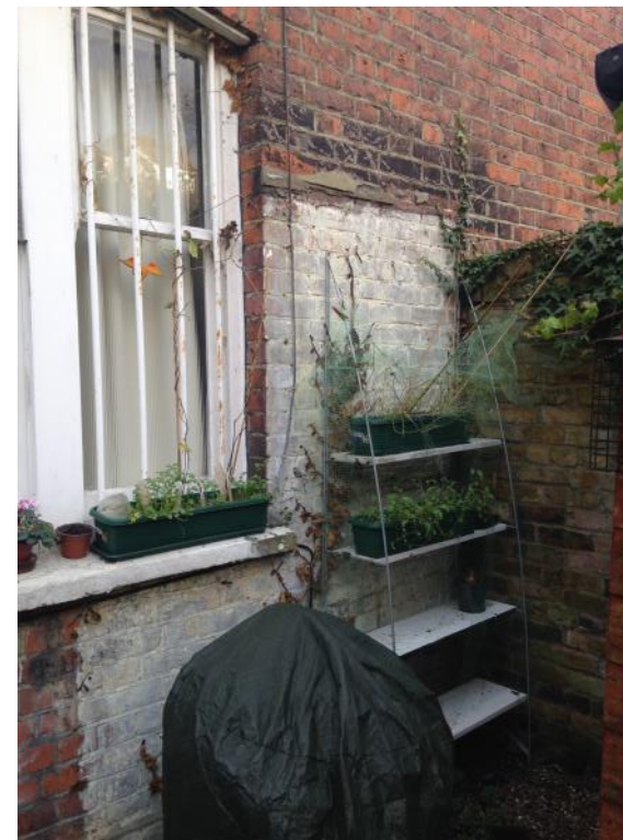
Figure 23: Detail showing the white painted brick section on the lower ground floor of No. 86 where there was once an extension.
