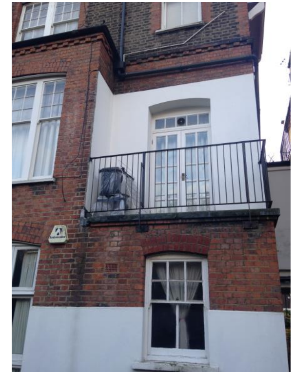
Figure 27: Detail showing the rendered treatment of part of the lower and upper ground floor of No. 88.
