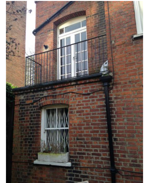
Figure 24: Detail of No. 86 showing the projecting lower ground floor and balcony at upper ground floor level.
