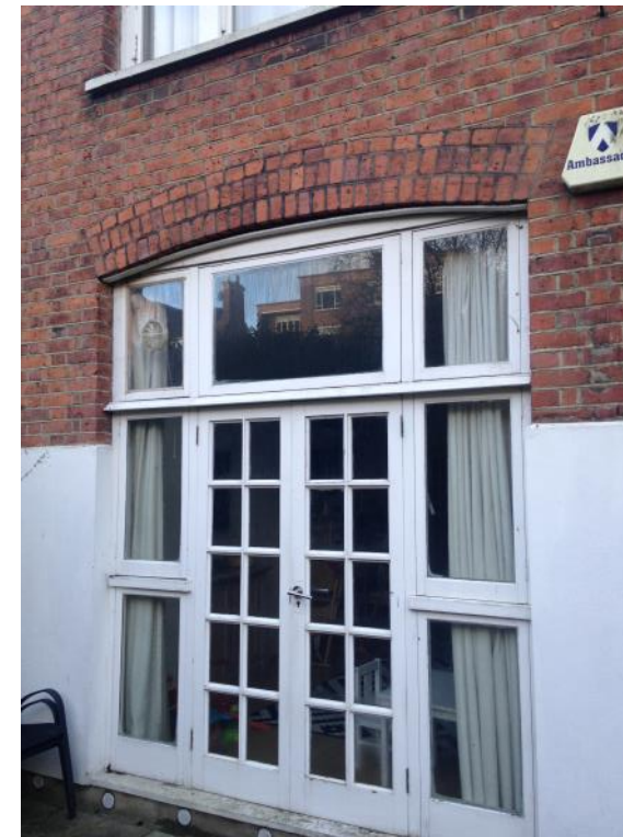
Figure 26: Detail of the rear door at lower ground floor level at No. 88. The treatment of the windows indicates that this opening was once a window that matched No. 86 (see Figure 22) but was extending to create a door.
