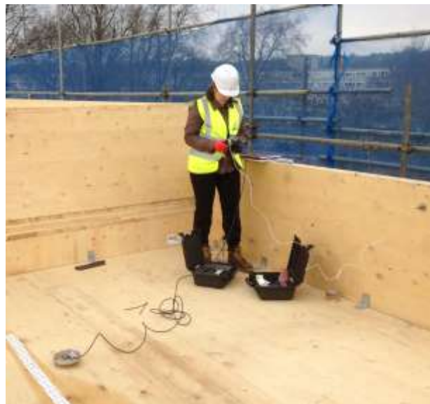
Figure 1: Vibration monitoring on CLT at first floor level and fourth floor level on the floor and wall
