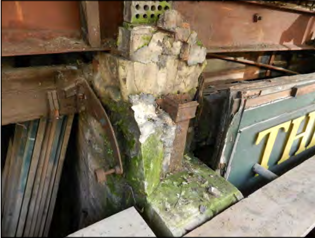
PH. N07. Natural Bath stone ground level pilasters. Stonework has been damaged by corroding embedded downpipes and inappropriate cement mortar repairs.
