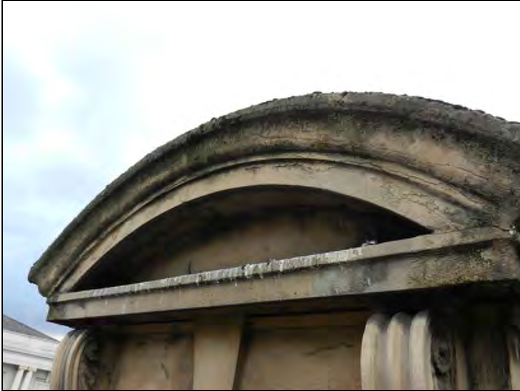
PH. N05. Curved pediment dormer window heads fractured and loose stucco, frost damaged brick and tile substrate. Take down and re-build new.
