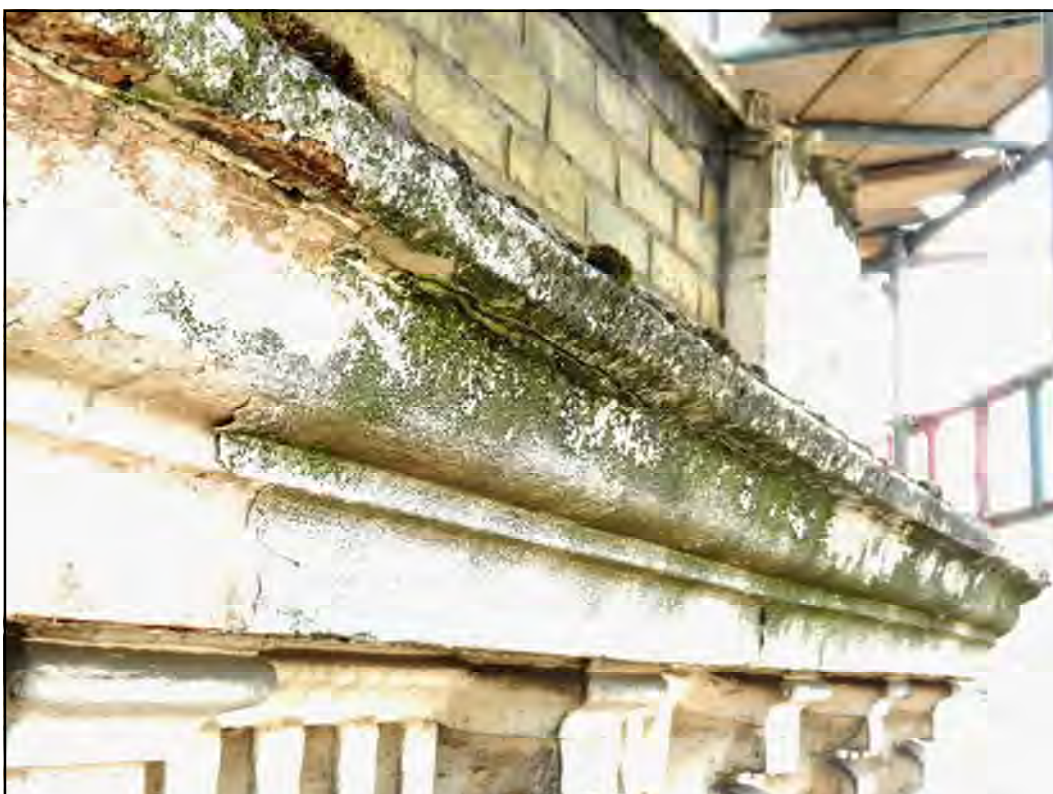
PH. N02. Cement mortar repair to upper cornice loose and de-bonding from the original substrate, continuous fracture through nosing. Remove complete and repair.
