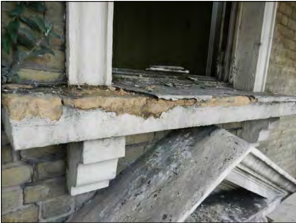
PH. N07. All natural Bath stone window sills cement mortar repaired. Repairs are loose and failing. Remove mortar and assess condition of exposed stone for most appropriate option on repair or replacement.
