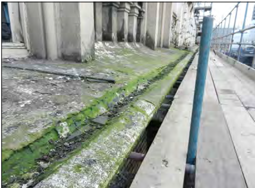
PH. N04. Original cornice detail with front gutter running to downpipe outlet. Flaunching below window sills and less built up to the base of balustrade.
