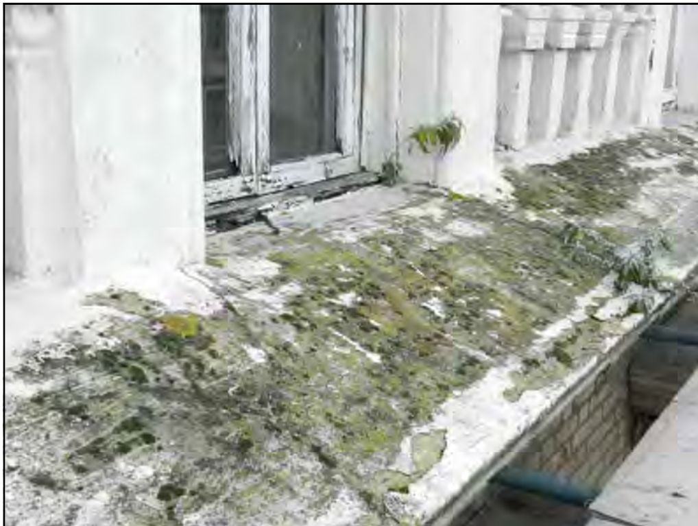
PH. S06. Cement mortar repair to lower cornice loose and de-bonding from original substrate, fracture through nosing, downpipe outlets blocked, weathering detail to window sills ineffective. Remove complete, repair substrate and revise weathering detail.
