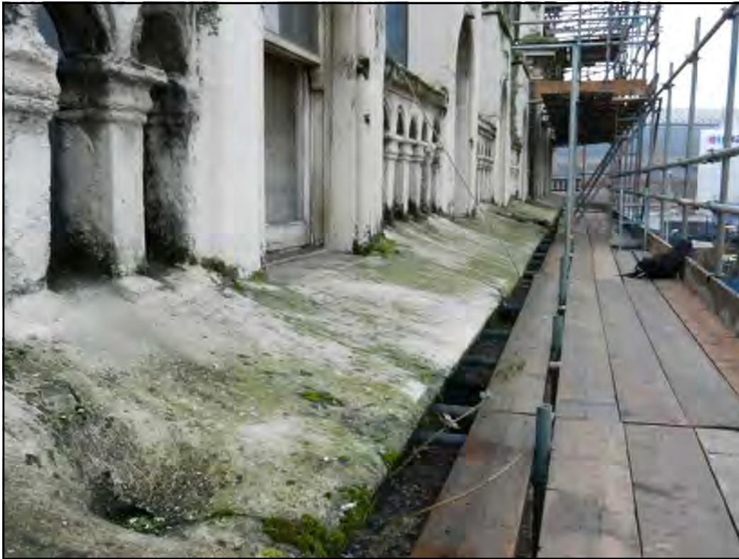
PH. N03. Cement mortar repair to lower cornice loose and de-bonding from original substrate, fracture through nosing, downpipe outlets blocked, weathering detail to window sills ineffective. Remove complete, repair substrate and revise weathering detail.
