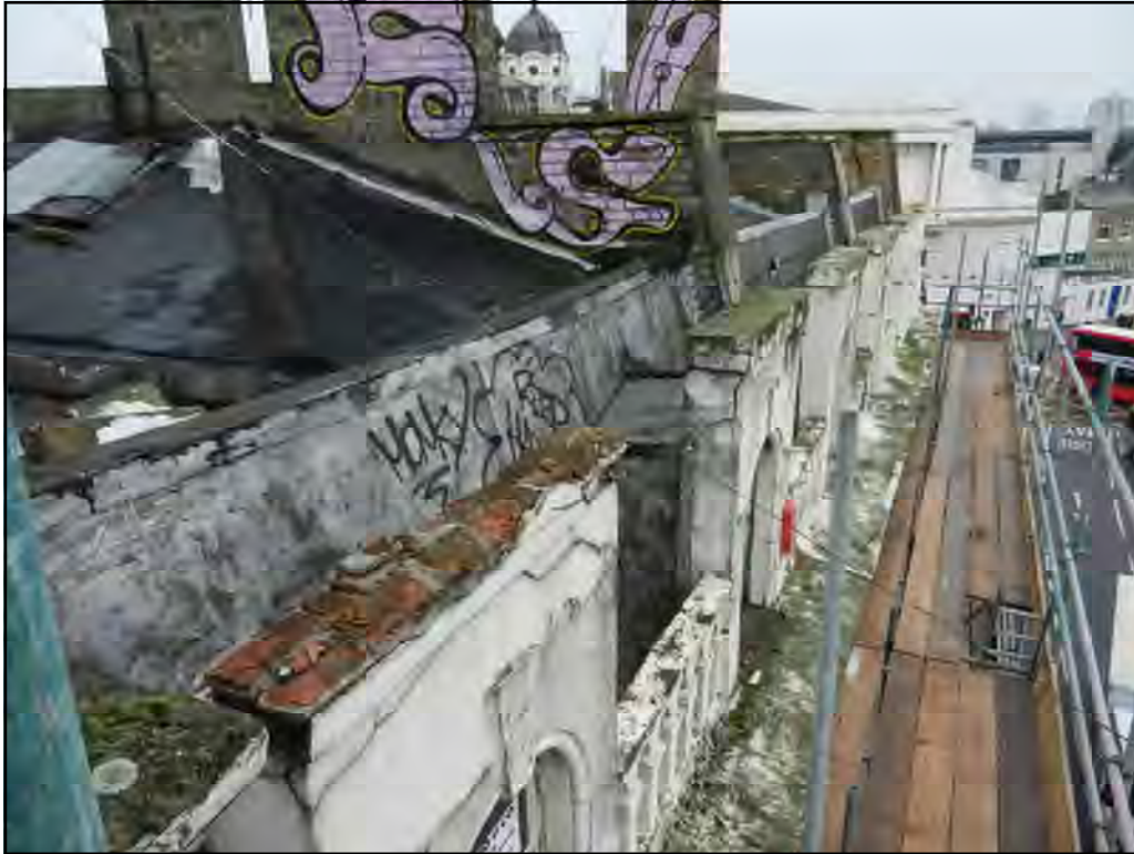
PH. S05. Dormer windows render loose and de-bonding, brickwork substrate frost damaged. Take down and re-build
