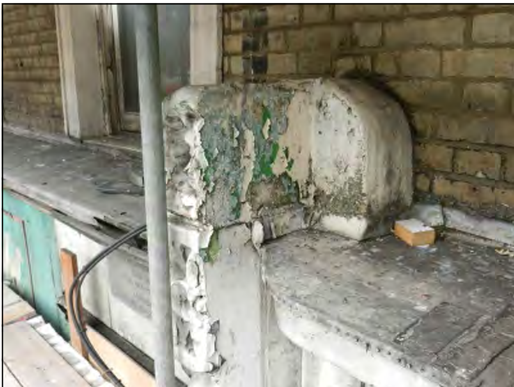
PH. N08. Natural Bath stone pilasters have been dramatically altered to accommodate previous change in shopfront. Remove and replace with new to match original carved detailing.
