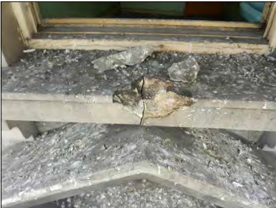
PH. N06. All natural Bath stone window sills cement mortar repaired. Repairs are loose and failing. Remove mortar and assess condition of exposed stone for most appropriate option on repair or replacement.
