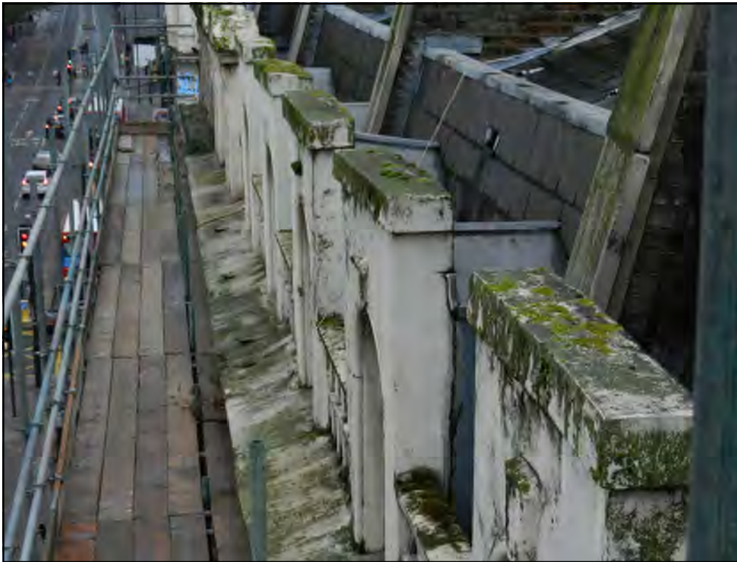
PH. N01. Dormer windows render loose and de-bonding, brickwork substrate frost damaged. Take down and re-build
