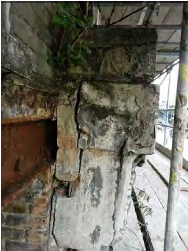
PH. N08. Top section of pilaster fractured and displaced. Carved detailing painted and mortar repaired.
