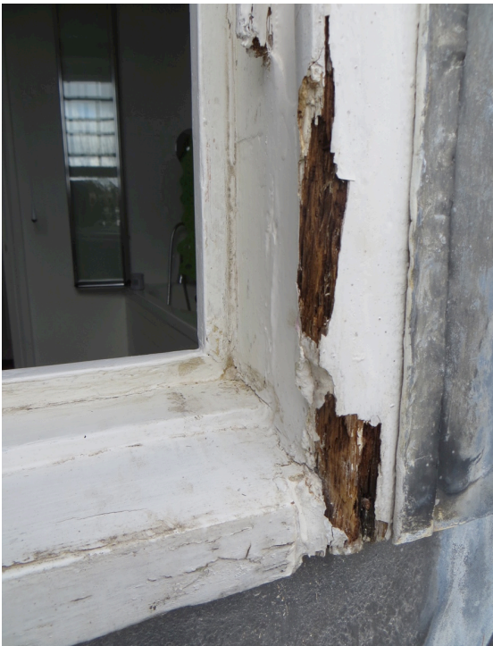
Figure 3. Photograph of rotten rear upper floor window.
