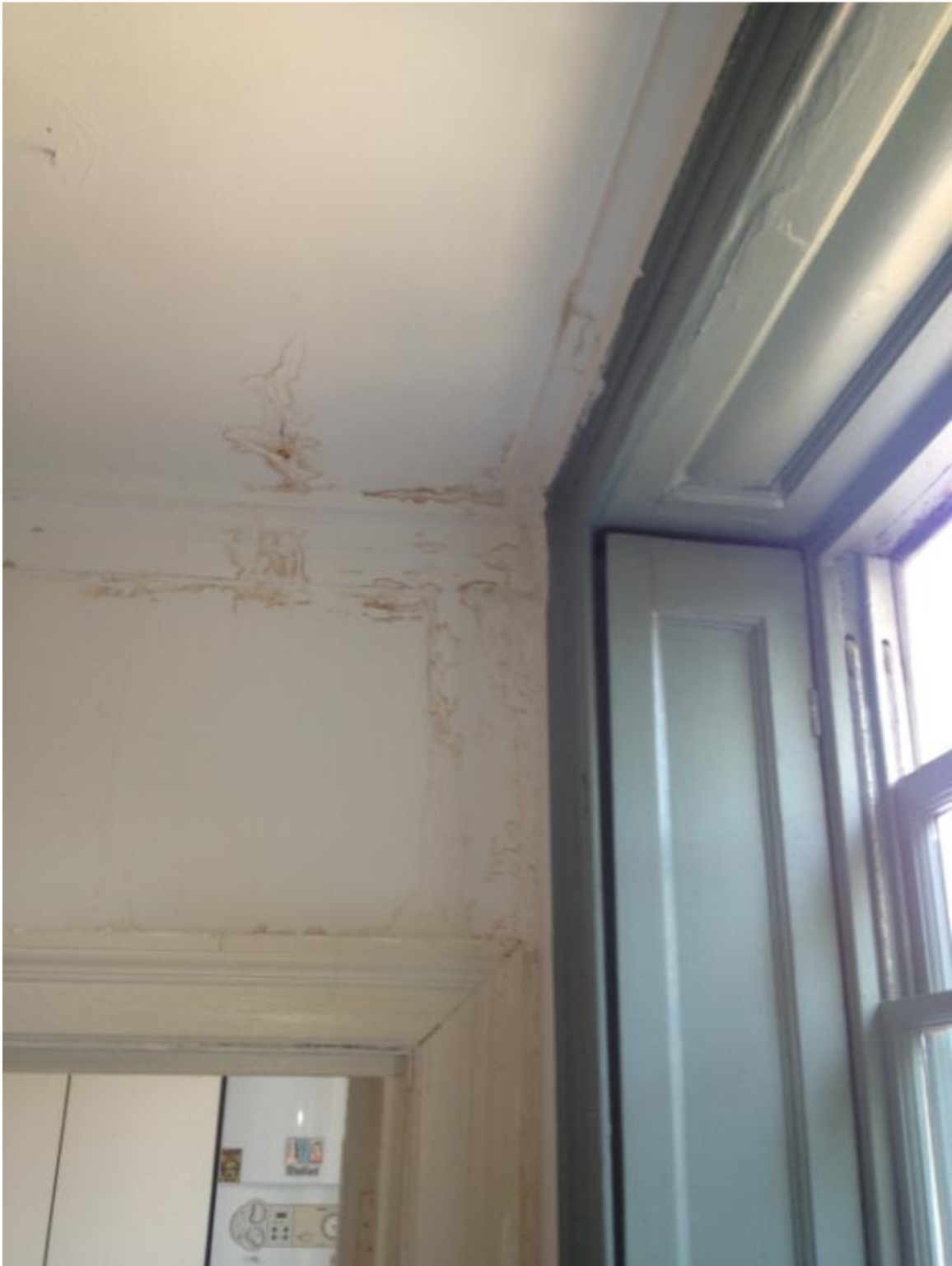
P4 Damp above rear window
