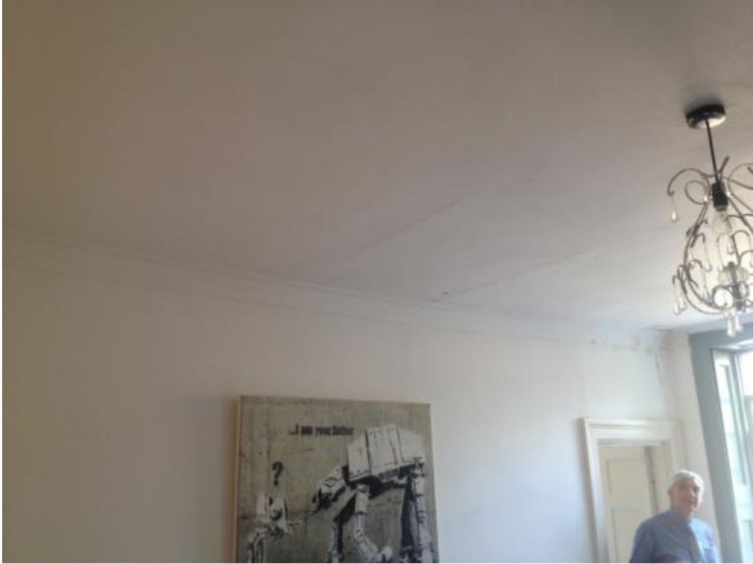
P5 Cracking to ceiling and bowing of cornice
