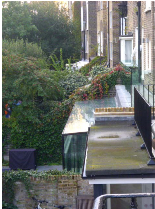
Precedent of glass balustrading at the neighbouring property no. 50 Regents Park Road at raised floor level on the rear terrace
