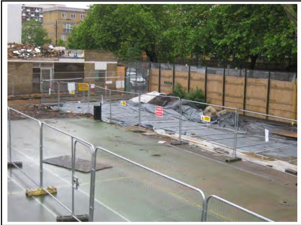
Area of asbestos contamination covered with plastic sheeting
