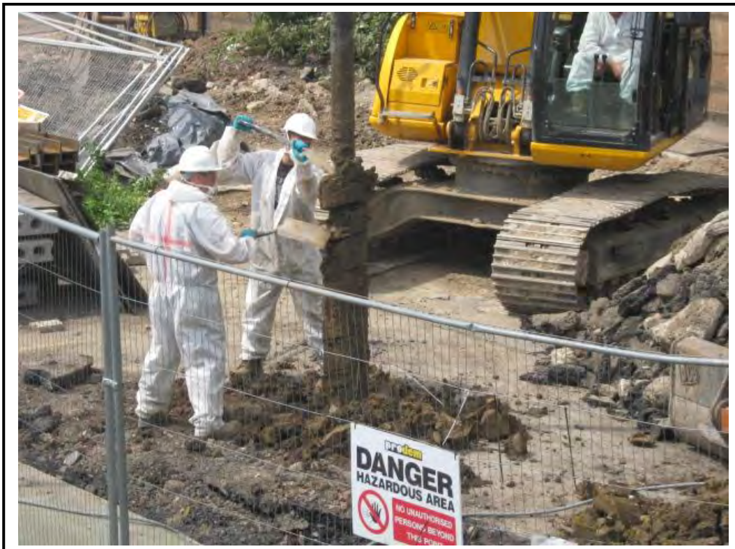
Piling through eastern limb may produce ACM containing soils beneath 1.5 m depth therefore we were informed that the pile arisings were dealt with as contaminated waste.
