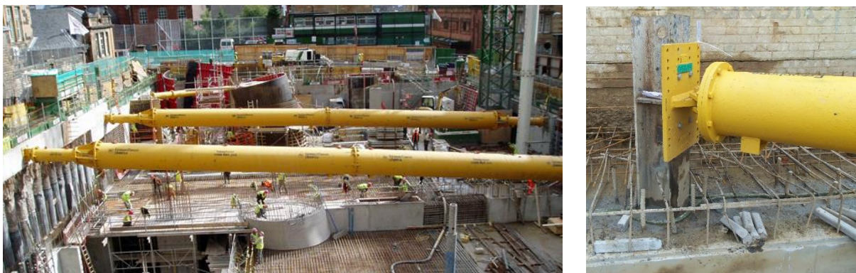
Figure 20 – Photo showing typical Groundforce struts spanning across a basement excavation © Groundforce & Figure 21 – MP125 Groundforce Strut End Plate Connection to Kingpost © Groundforce
