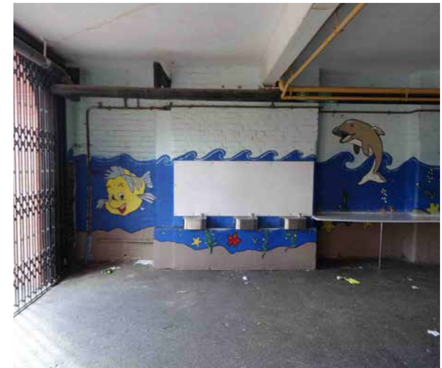
Fig 4.10 Painted walls in the undercroft are to be removed by non-abrasive means or overpainted.
