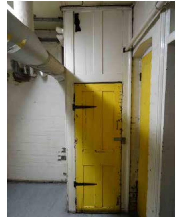
Fig 4.6 The lift enclosure and door proposed for removal. The door appears to be a later addition as it is poorly fitting with ad hoc hinges.
