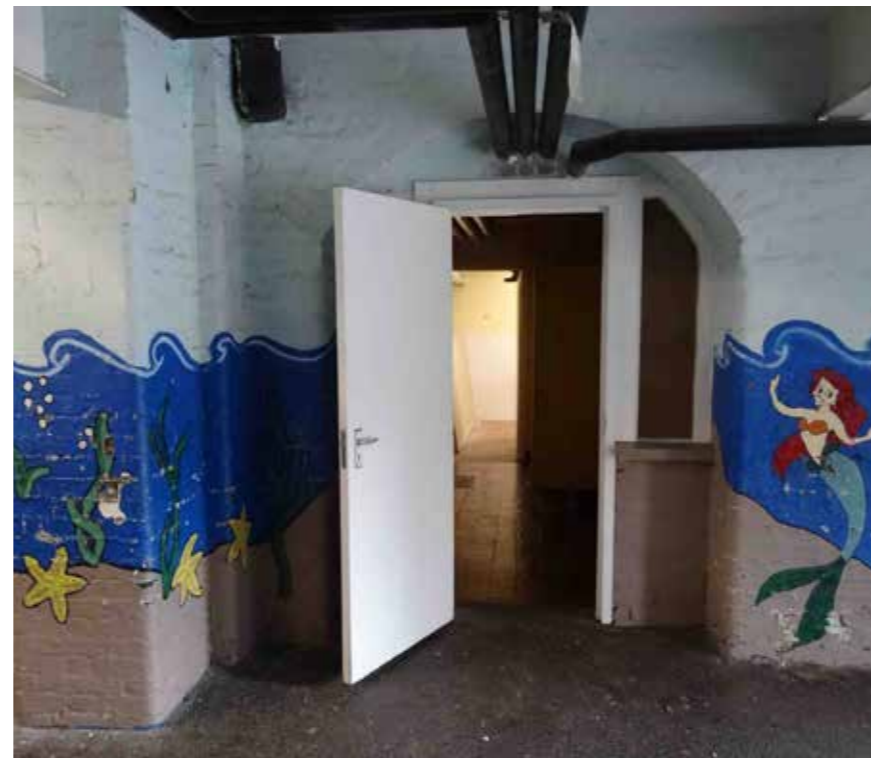
Fig 4.9 Painted walls in the undercroft are to be removed by non-abrasive means or overpainted.
