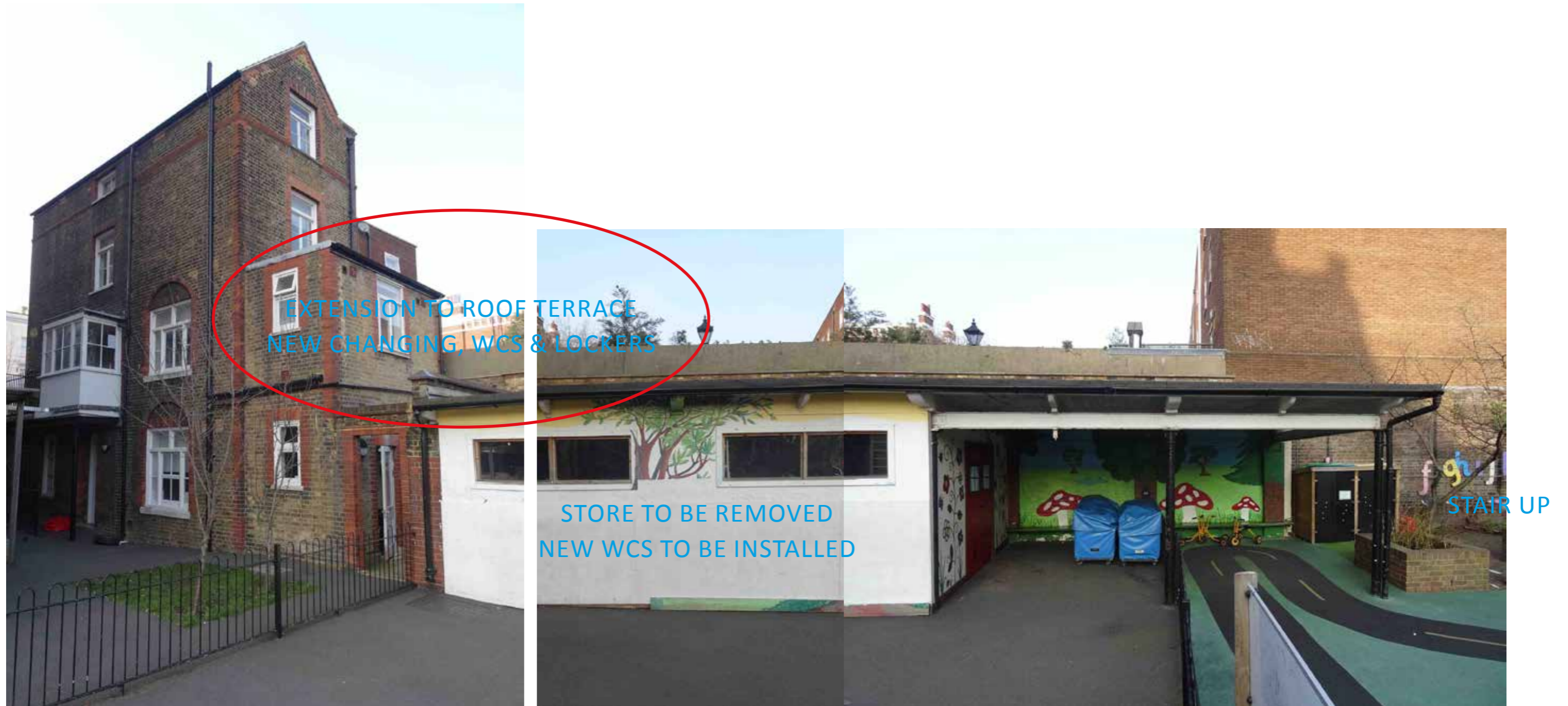
Location of proposed rear extension to the rear of the Caretaker's house.
