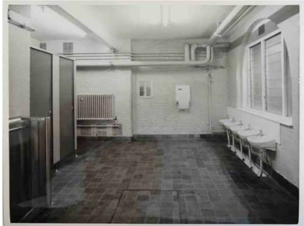
Fig 3.9. Photo of the Junior Boys toilet in 1971. The room has been sub-divided since.
