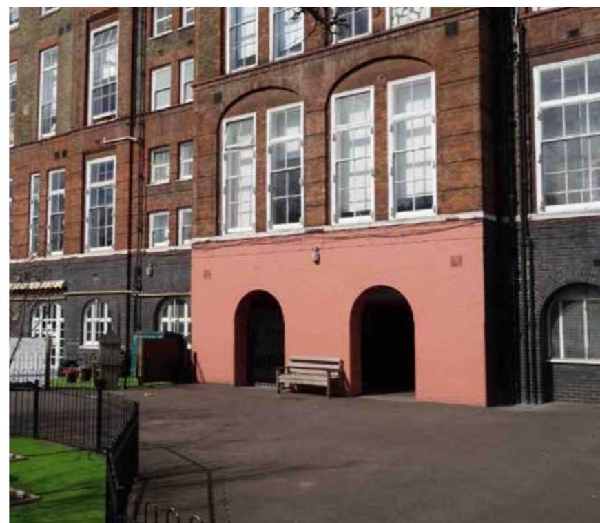
Fig 4.11 The paint on the exterior wall by the Buffer Space is to be removed by non-abrasive means.
