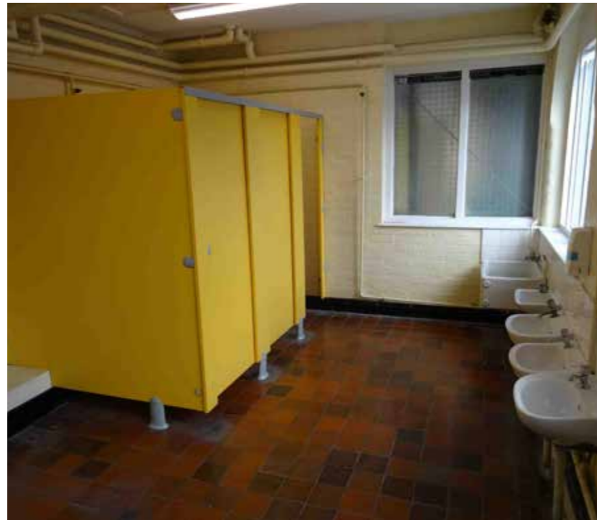
Fig 4.5 A recent photo of the undercroft WCs. The fixtures, floor and brick partition walls are to be removed.
