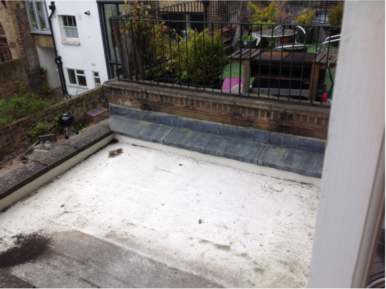
Photo 1: View of existing flat roof of no.44 Chalcot Road from first floor kitchen, showing how it abuts terrace at 43 Chalcot Road
