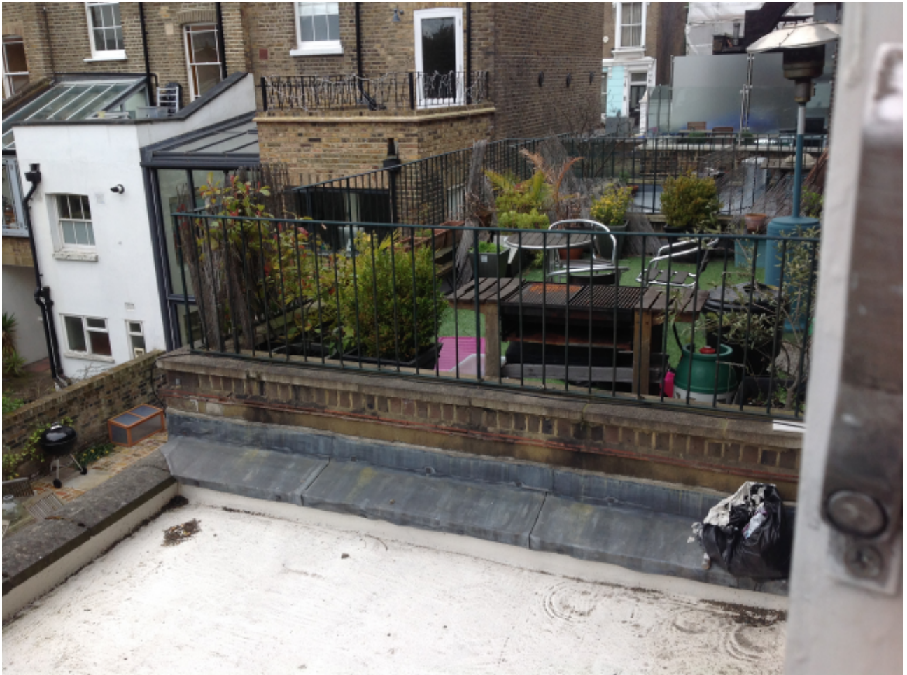
Photo 5: Flat roof of no. 44 Chalcot Road and adjacent terrace at no. 43 Chalcot Road
