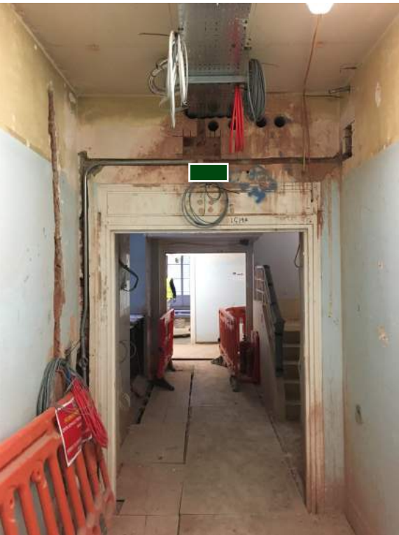
Above Door wall mounted
