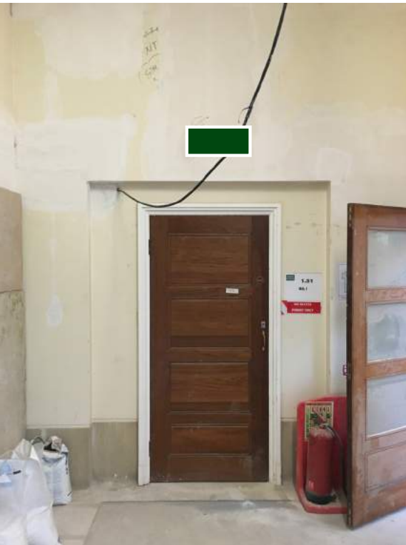
Above Door wall mounted
