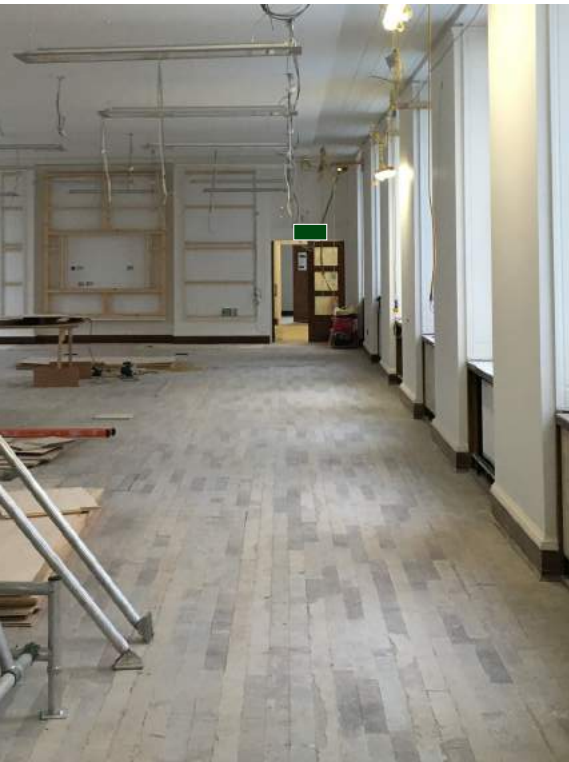
Above Door Wall mounted
