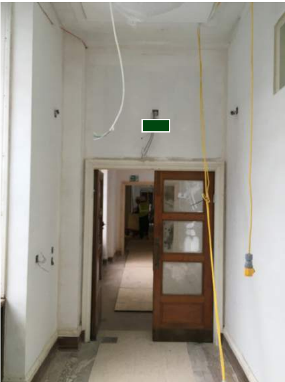
Above Door wall mounted
