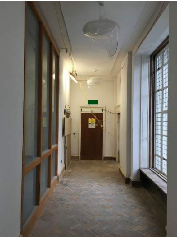
Above Door wall mounted
