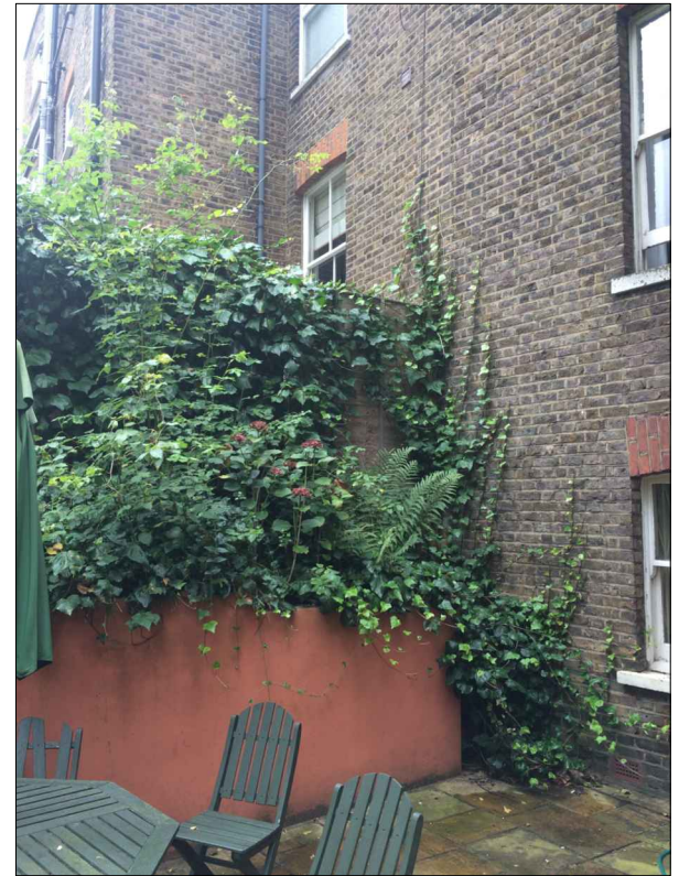
EXISTING MASONRY AND TIMBER GARDEN WALL ON A BOUNDARY WITH NO 23 KINGDON ROAD, APPROX HEIGHT 3.6M
