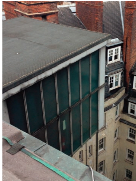
Existing Lift Motor Room
