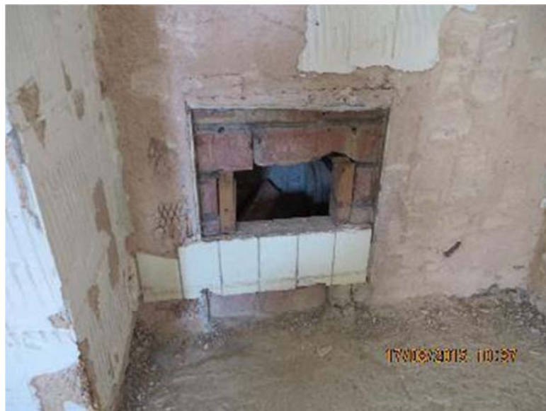
Figure 3-4: Typical holes/cracks/crevices in brickwork observed during the internal inspection.
