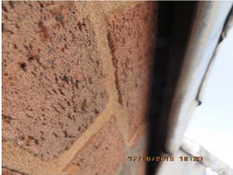
Figure 3-3: Gap where lead flashing meets the brick wall on the roof providing potential roost for bats
