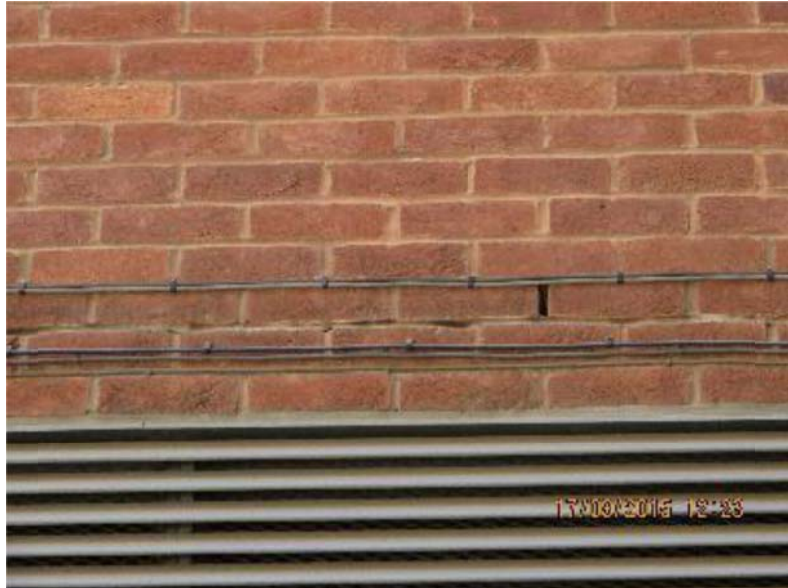
Figure 3-2: Weep holes in brickwork leaving crevices provide potential roosting and/or access for bats
