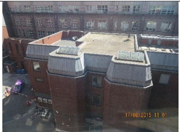
Photograph 6: Roof of eastern arm of the building, taken from inside the western section
