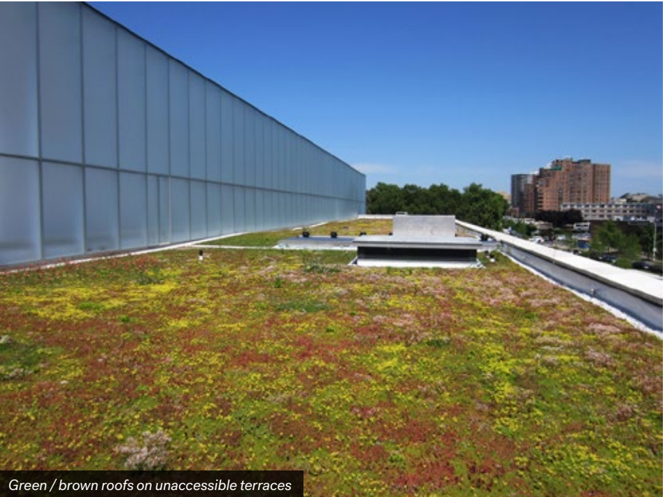
Green / brown roofs on inaccessible terraces
