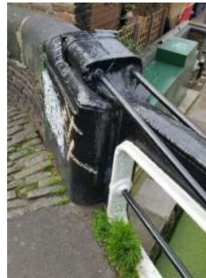
The listed cast iron bridge structure forms a key focal point and boundary to the site
