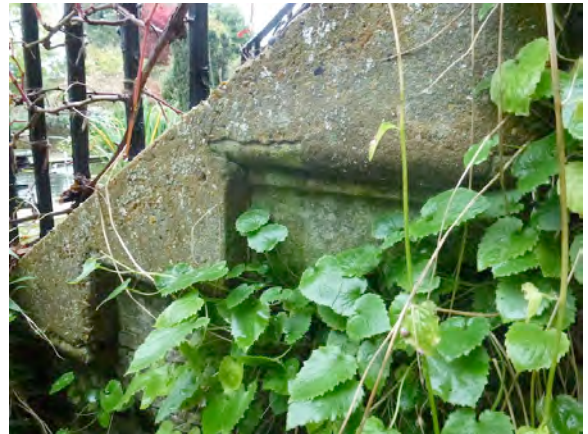
Details of stone staircase with wrought iron balustrade; note concrete capping to profiled stonework
