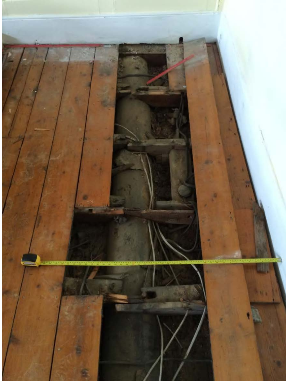
Photo 25 – Poor connection of joists on to North-West 2 nd floor bressummer
