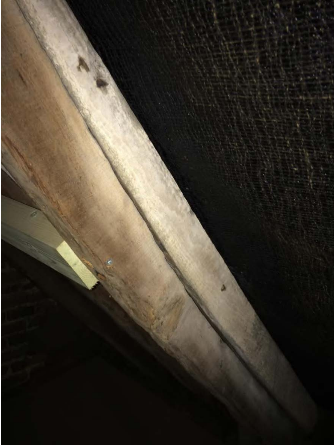
Photo 5 – Significant firrings to correct sagging rafters
