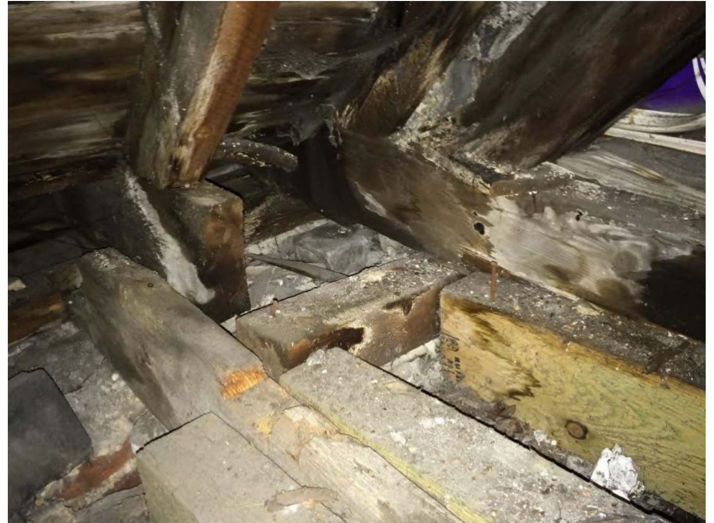
Photo 24 – Significant water staining to rafter ends within rear eaves. Cut truss chord.
