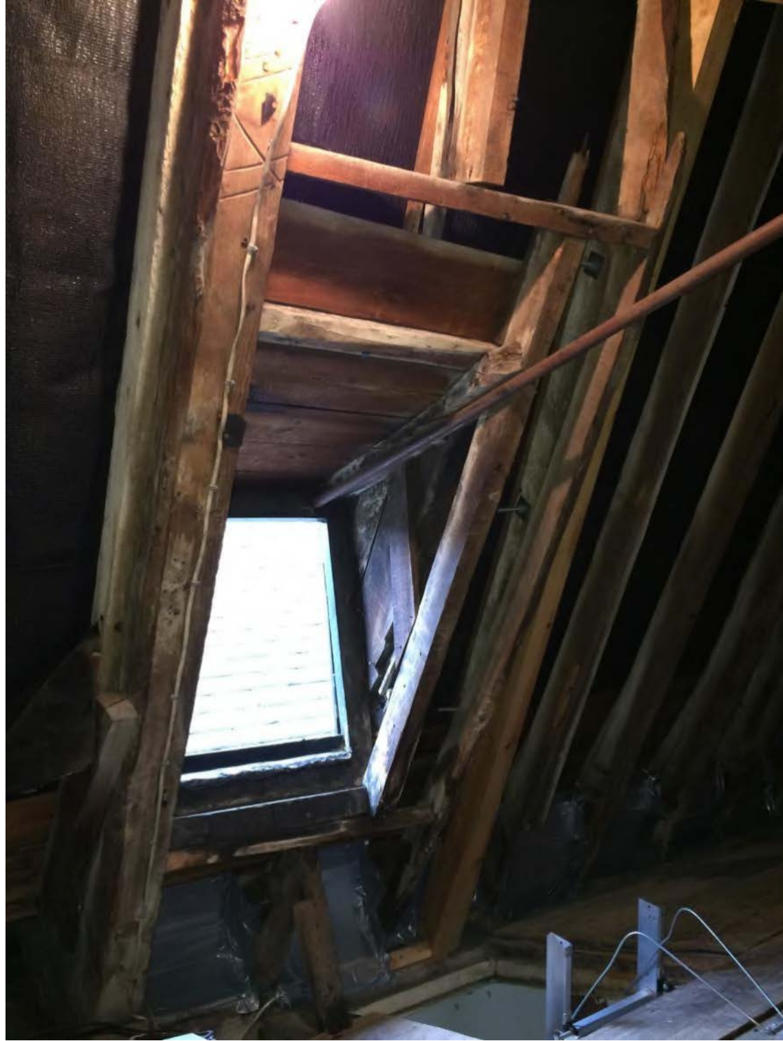
Photo 9 – Fracture to roof hatch trimming timber on right hand side
