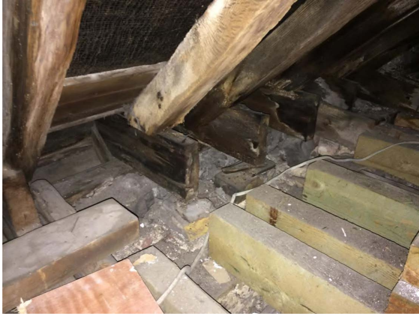
Photo 21 – Loss of connectivity between rafter ends and second floor joists. Existing joists appear to have been severed.
