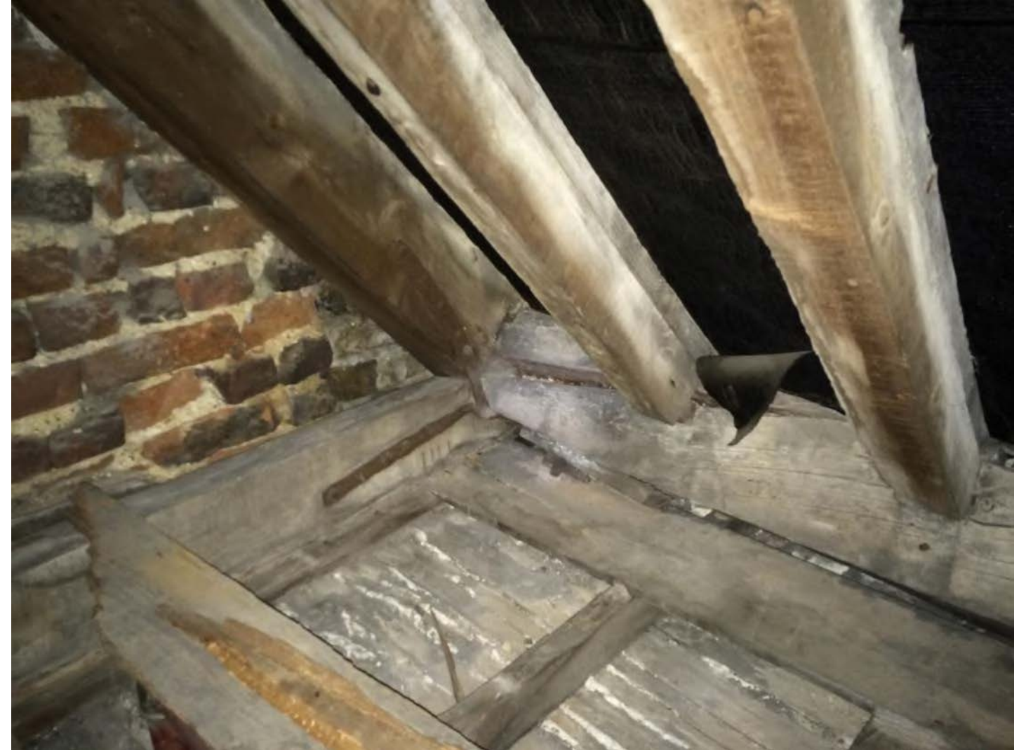
Photo 12 – Fractured purlin at tenon connection with northern principal truss
