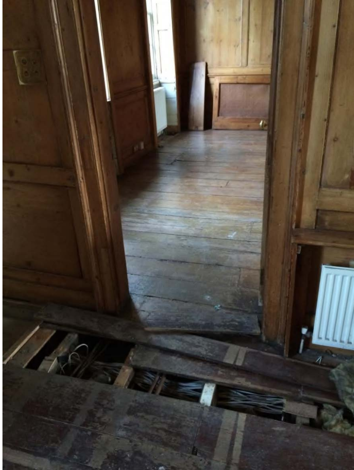
Photo 29 – Sloping floor to East-West central spine wall at upper ground floor level
