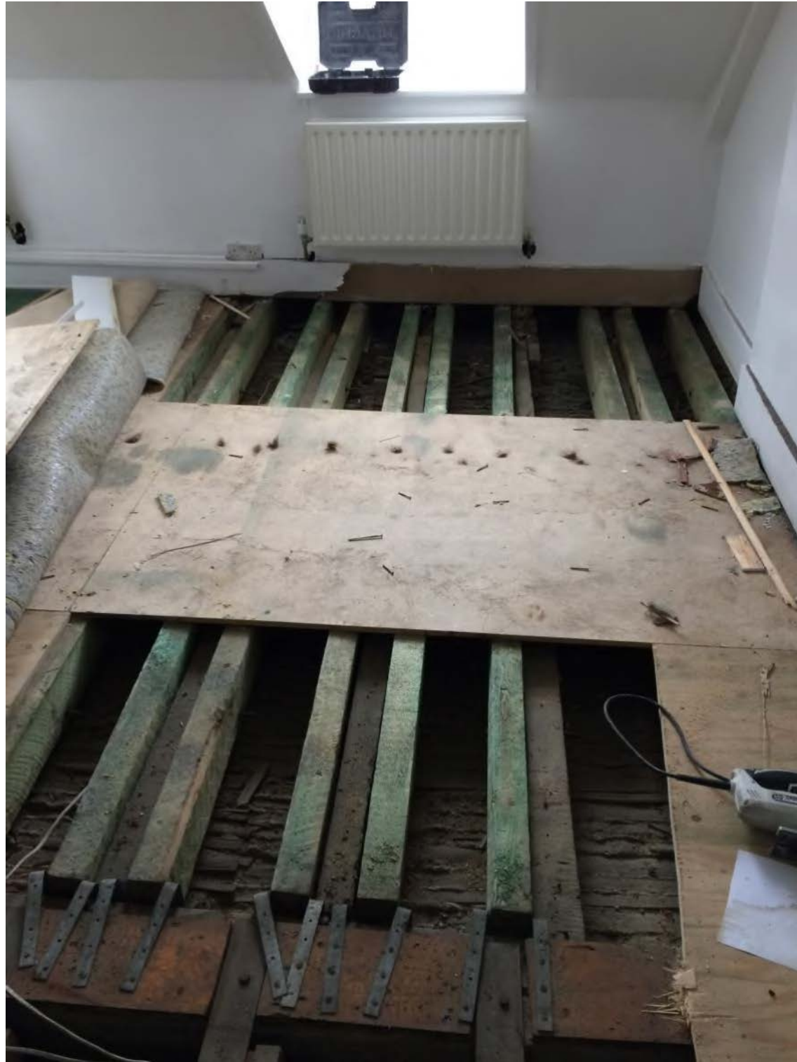
Photo 23 – Supplementary modern timbers installed either side of existing joists and poor detail over bressummer
