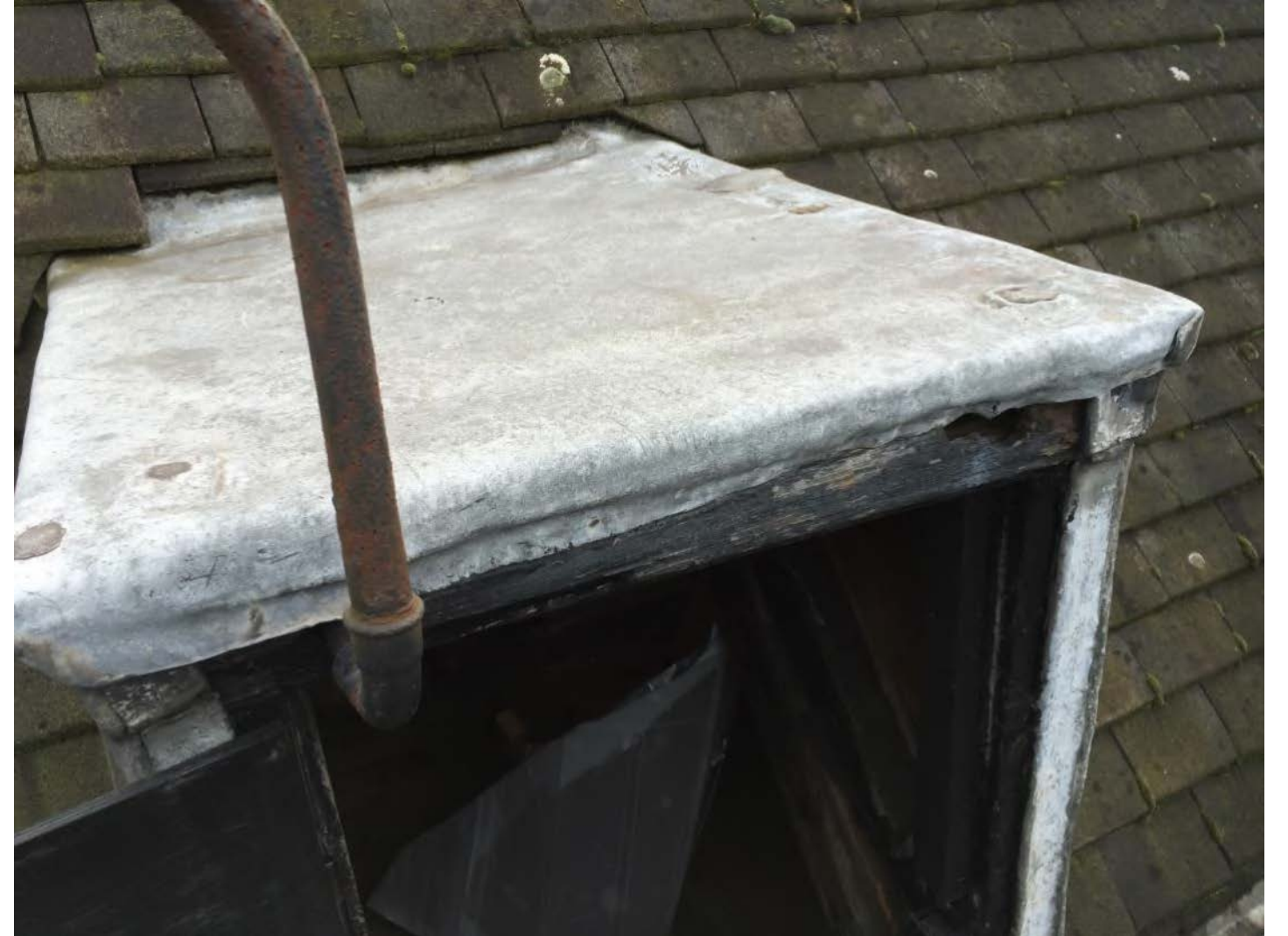
Photo 6 – Decaying timber surround to roof hatch
