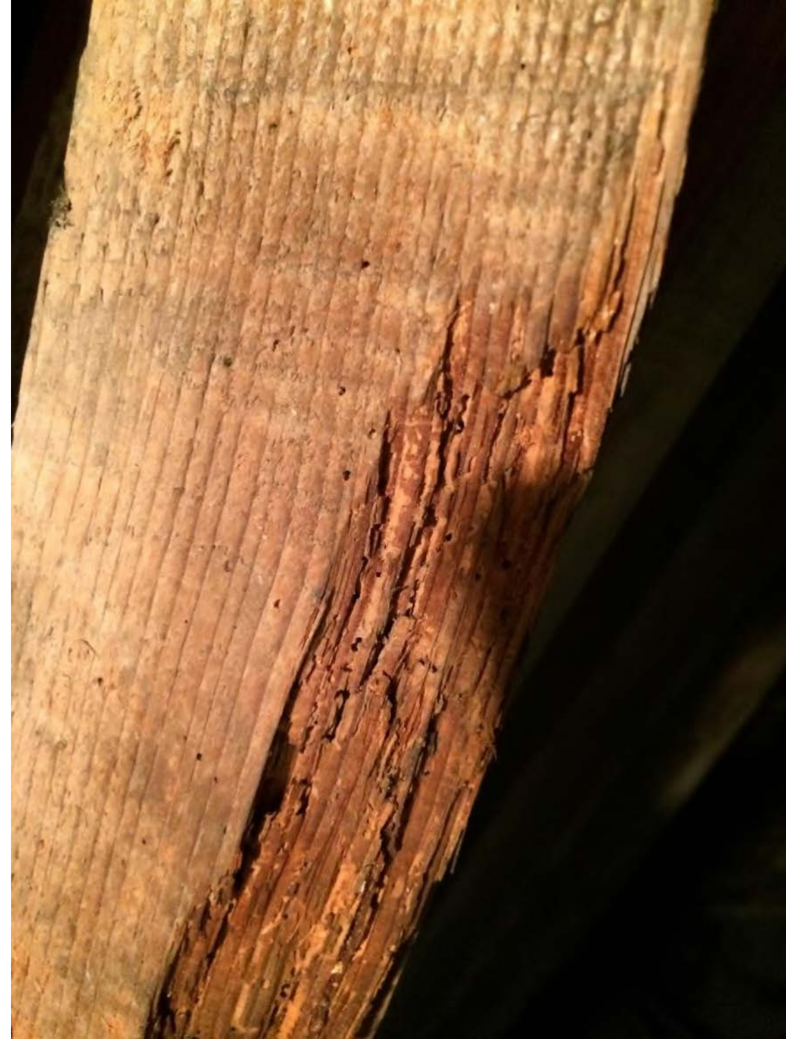
Photo 16 – Insect bores to timber rafter
