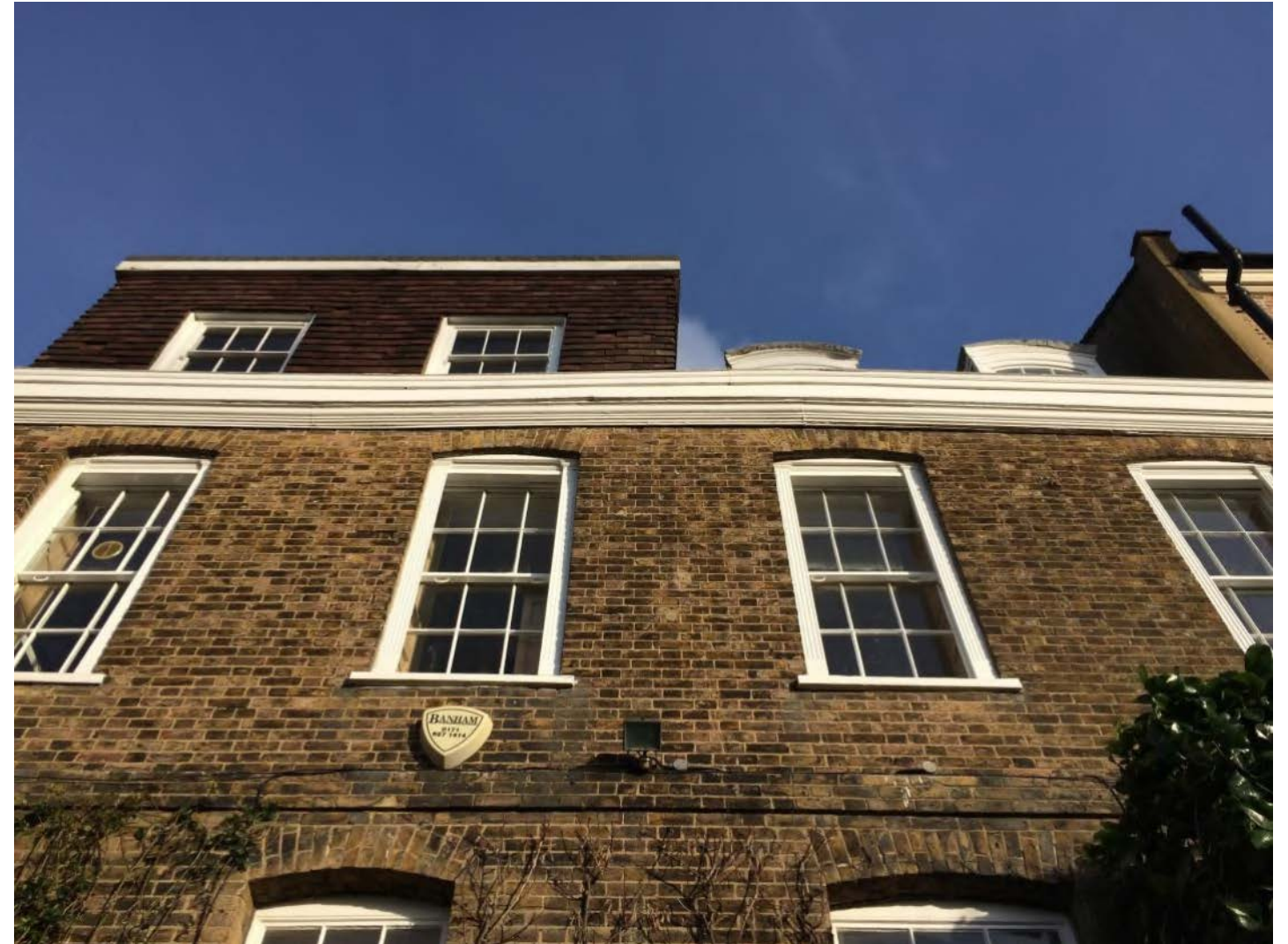
Photo 20 – Bowing of rear elevation at mid-point of 2 nd floor level
