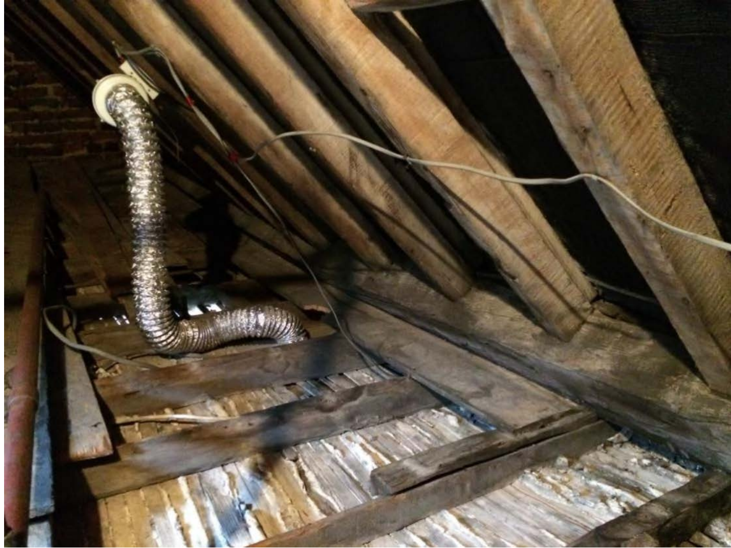
Photo 15 - Significant deflection of North-East purlin
