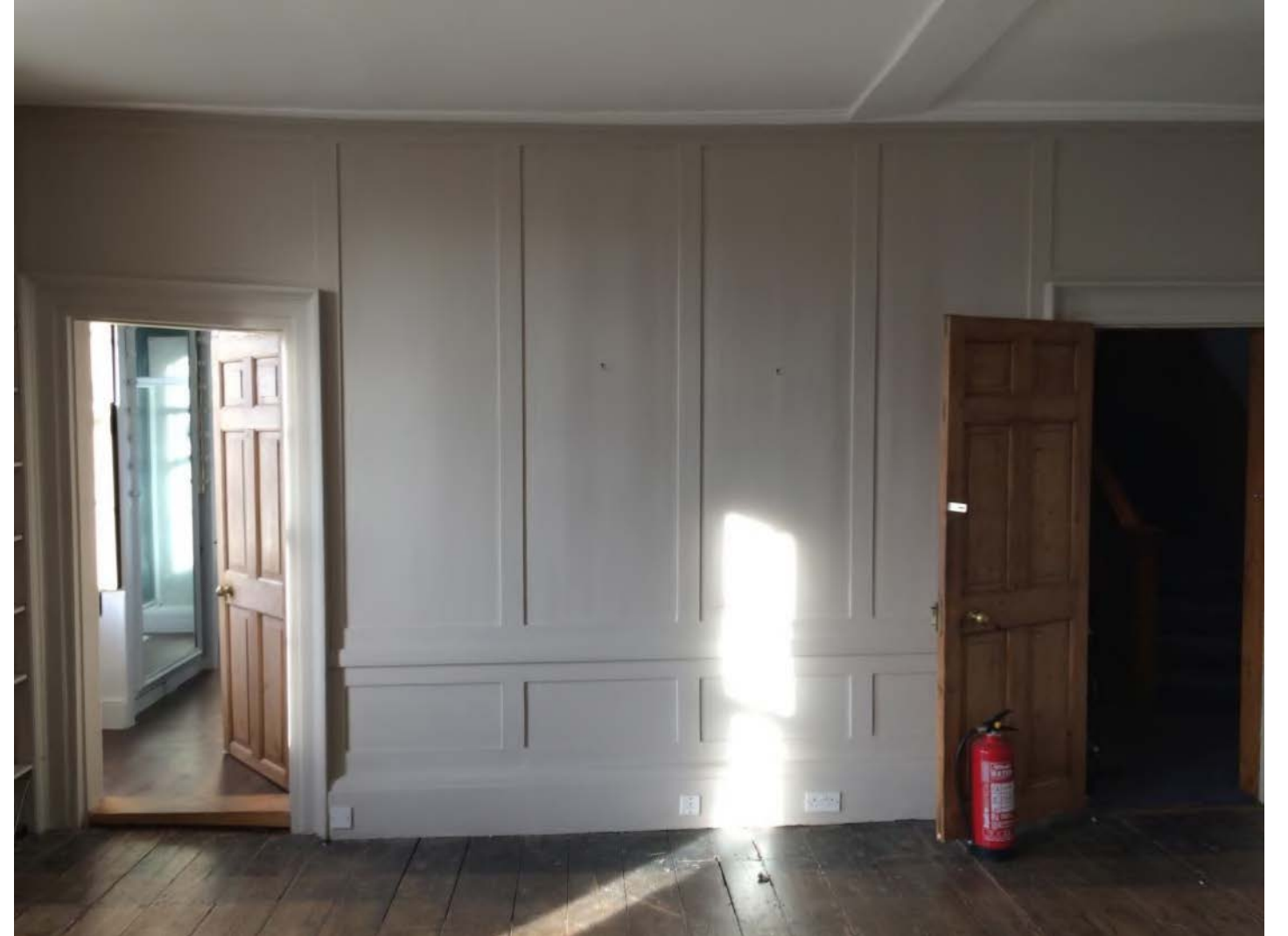
Photo 26 – Sloping floor and lozenging of doors in Bedroom 1 at 1 st floor level
