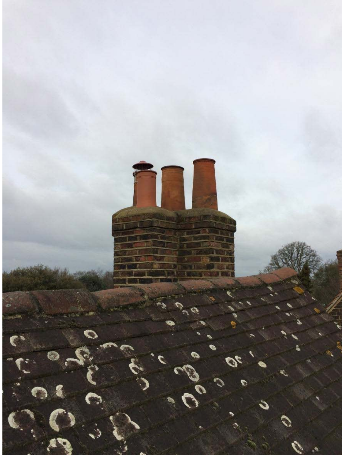
Photo 13 – Flaking surface to clay pot
