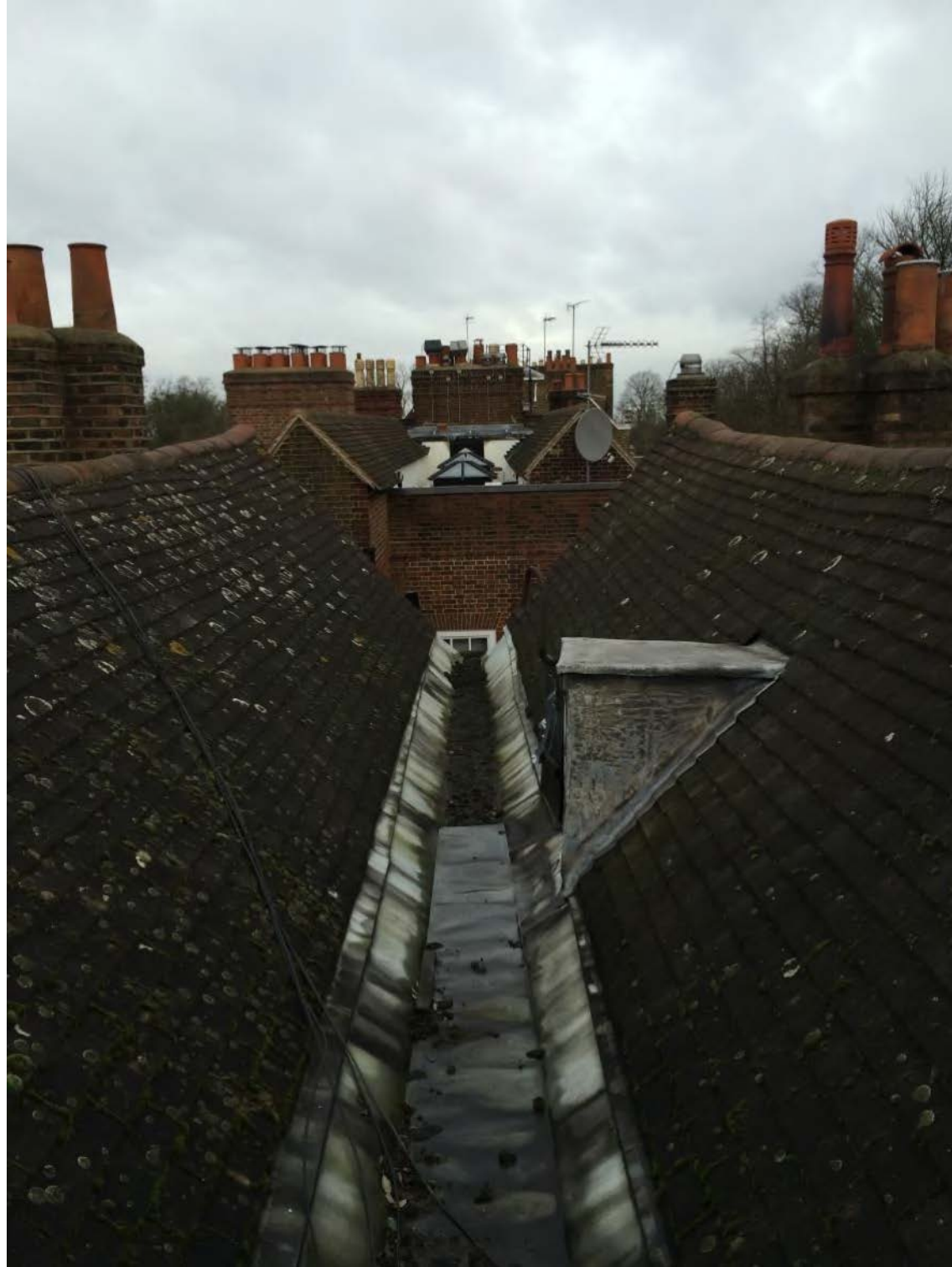
Photo 11 – Silting of valley gutter
