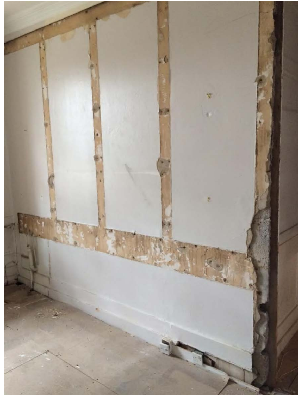
Photo 28 – Sloping floor to modern blockwork partition
