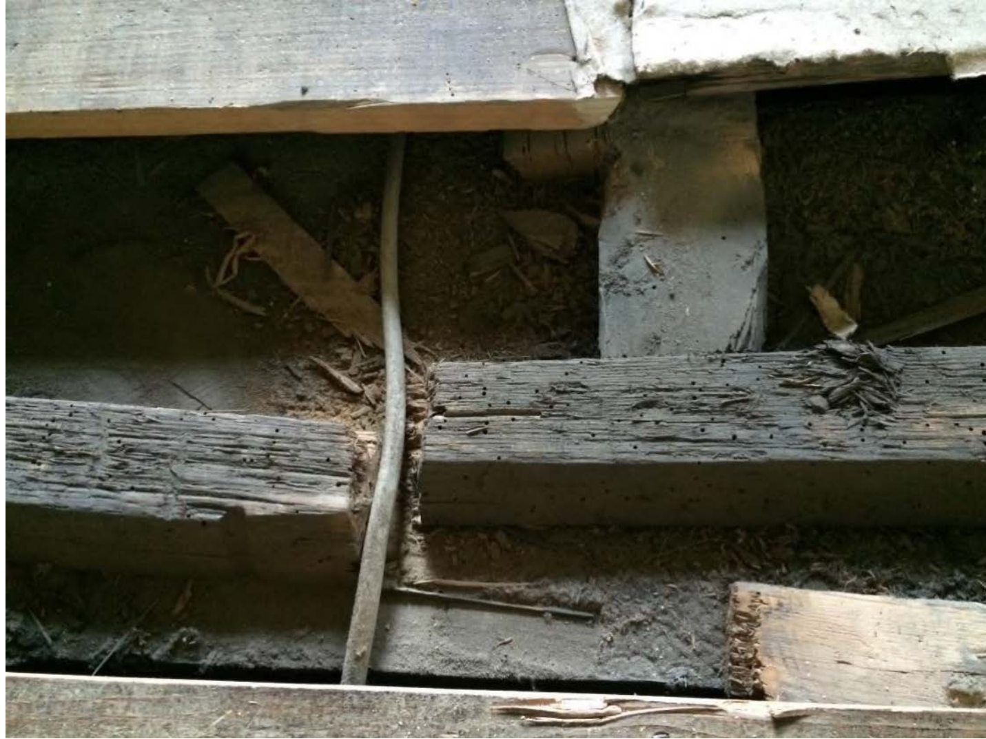
Photo 17 – Insect bores to timber floor joist and heavy notching of battens
