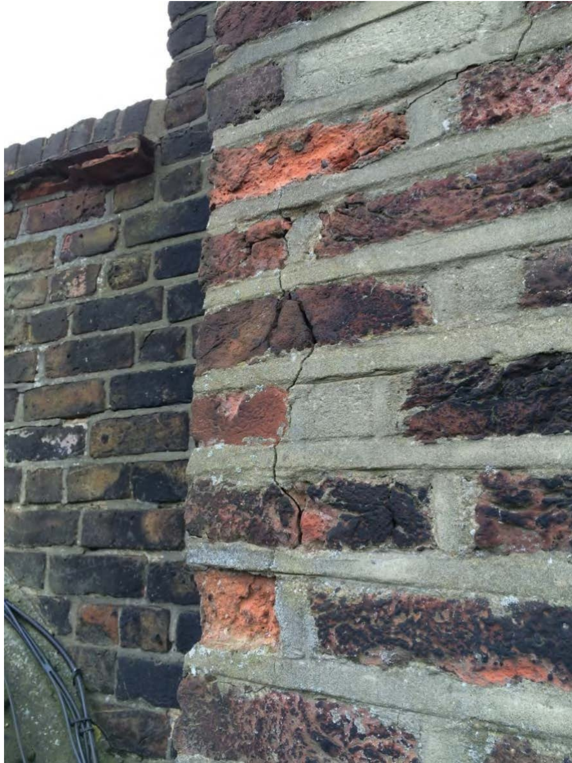
Photo 3 – Blown face of brickwork and vertical cracking to northern face of southern stack
