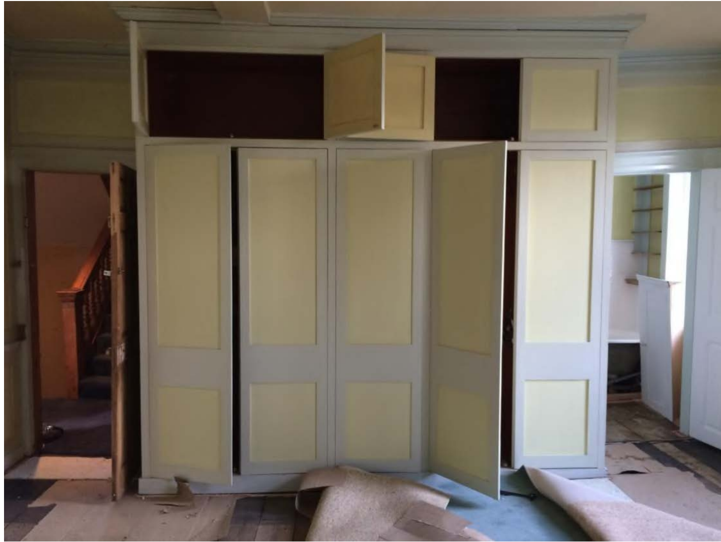
Photo 27 – Sloping floor and lozenge of doors in Bedroom 2 at 1 st floor level
