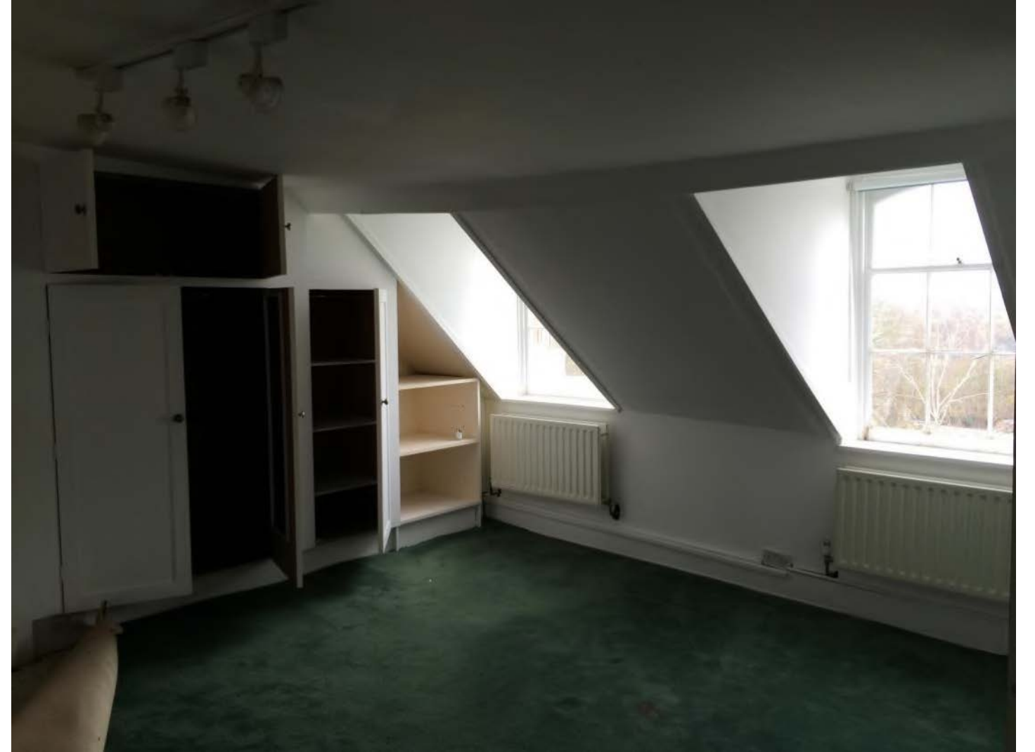
Photo 14 - Significant deflection of South-West purlin
