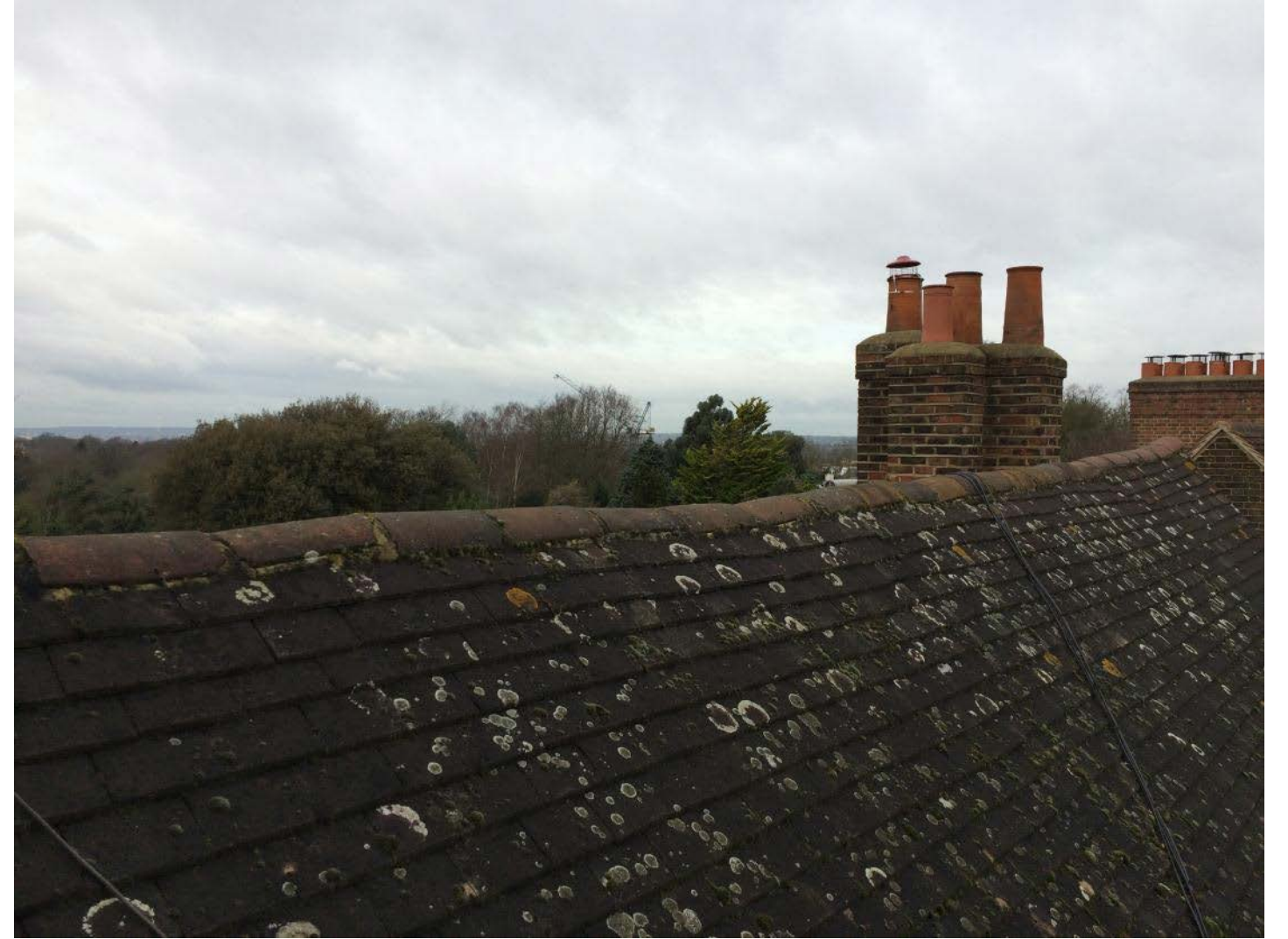
Photo 10 – Minor sagging of roof pitch
