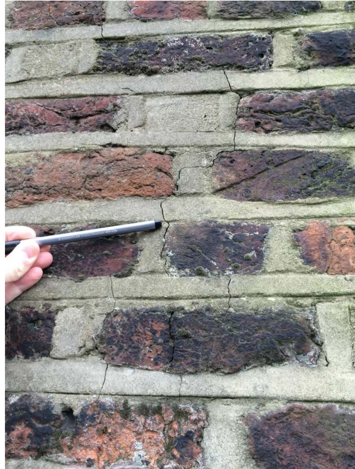
Photo 2 – Vertical crack in face of southern stack
