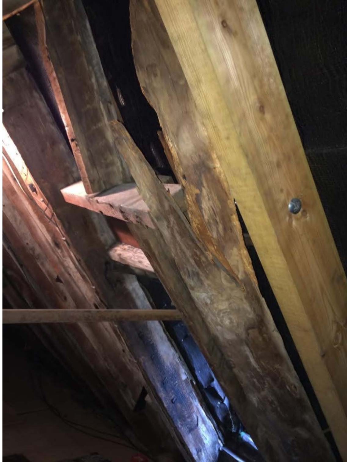
Photo 7 – Fracture to roof hatch trimming timber
