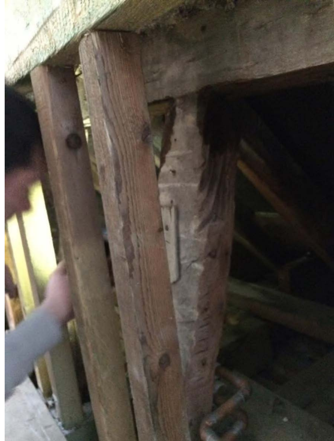
Photo 22 – Original dwarf stud walls leaning to rear elevation behind modern corrected wall line
