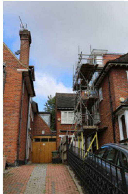
right 80 Lawn Road - nine pane stair window and dormer bay, under construction two storey garage wing left 81 Lawn Road - nine pane stair window and dormer bay gabled brick garage wing with dormer level
