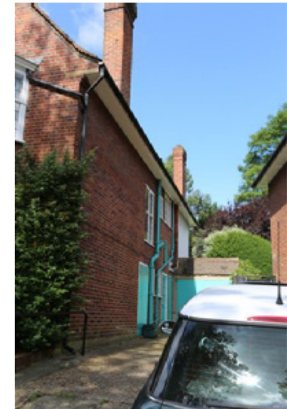
77 Lawn Road - subject site four panel stair window later addition precast concrete garage
