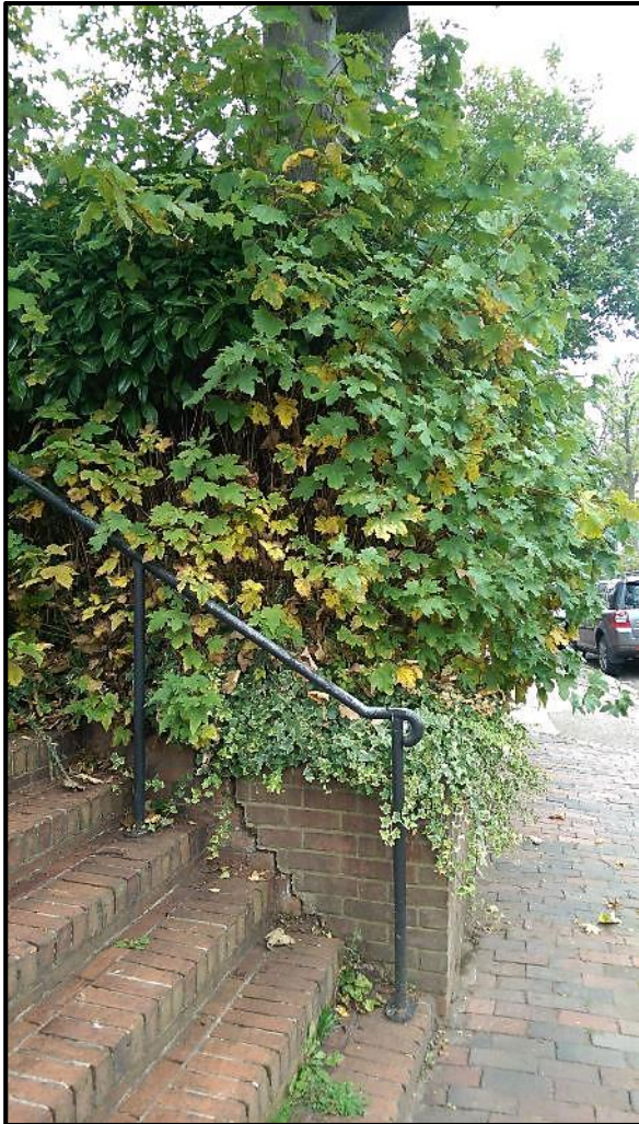
Plate 11. The base of T10 as viewed from Lawn Road, looking north. The dense sucker growth is visible, together with the diagonal crack in the retaining wall next to the steps.
