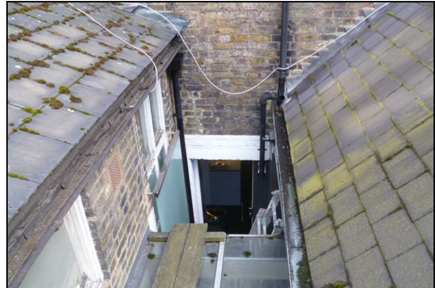
Fig 10. Photo to show the shared lightwell to the rear of the building.
