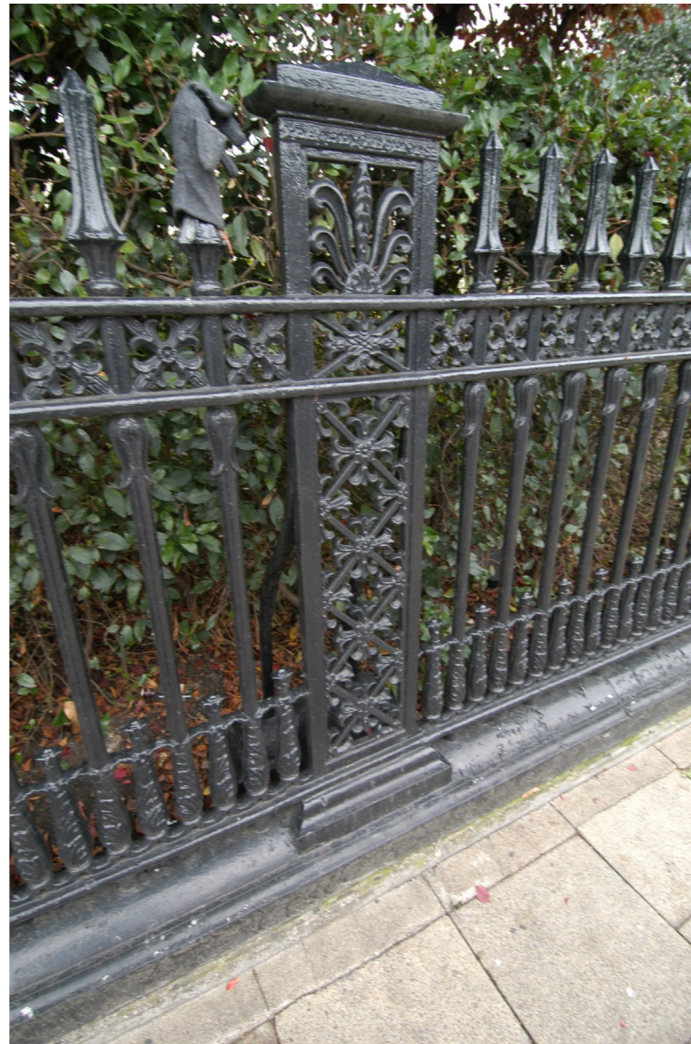
Photo no. 13 Flat front standard with backstay Listed Railings RL15 (part of EH list entry no. 1244298)
