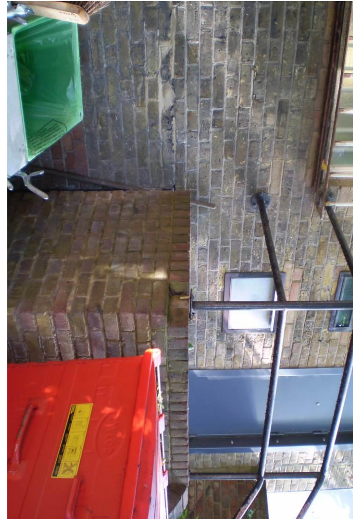
Plate 14 – Crack damage to the step beyond the area of N° 171A (with gap between wall and step structure)
