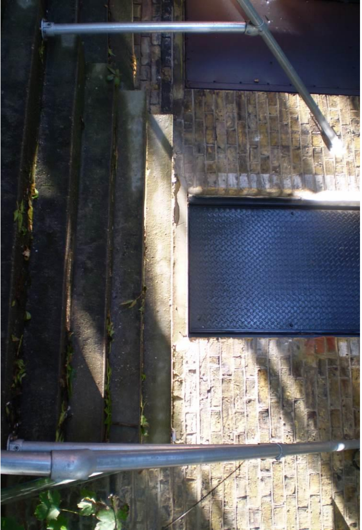
Plate 17 – Damage to threshold at the top of rear steps to adjoining property
