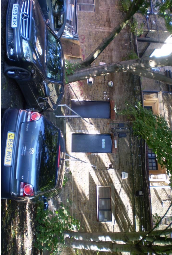
Plate 1 – General view of the rear area of the Basement to N° 171A and adjoining property
