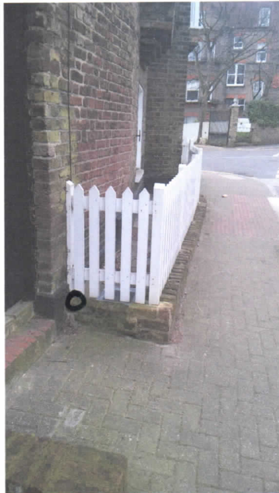
Figure 4: Outfall onto pavement
