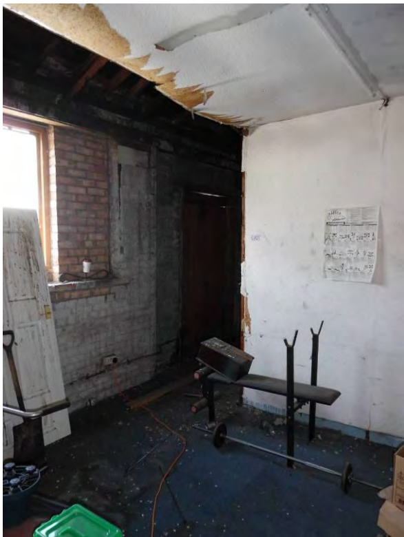
Fig.29 First floor partitioned space at the front of the building looking south east
