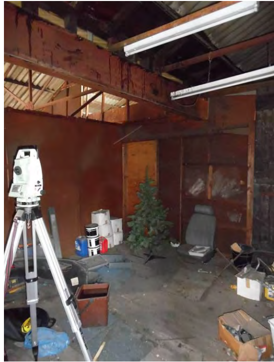
Fig.32 First floor part partitioned space at the front of the building looking north east
