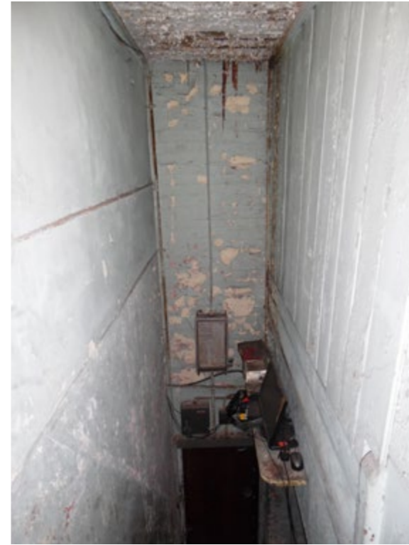
3. Damp within First Floor Stairwell
