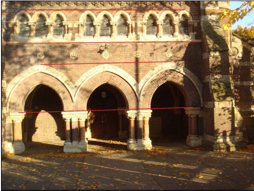
Plate 5. Narthex showing settlement of column right of centre and negligible effect on alignment of wall above.
