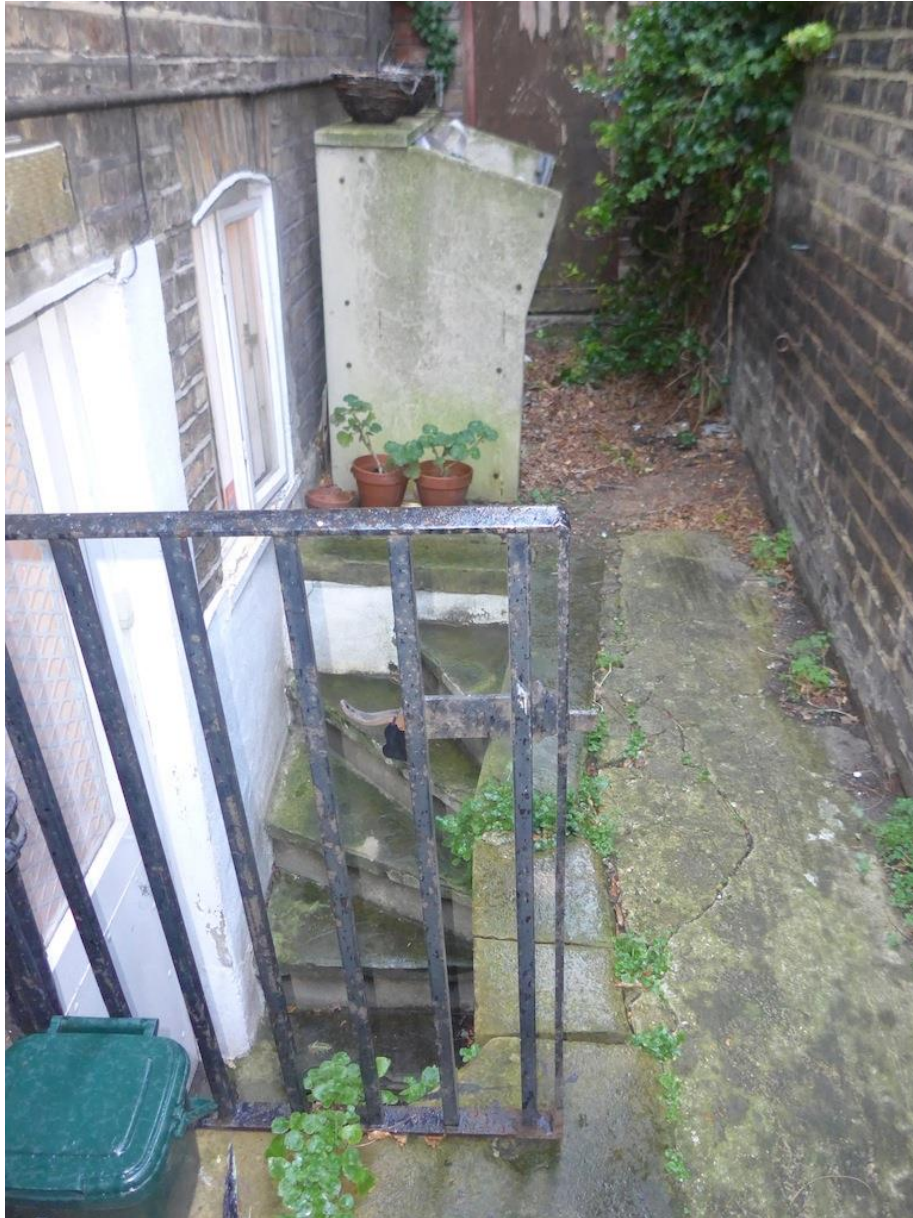
Photograph 2. Detailing the side passage and steps to the lower ground floor level
