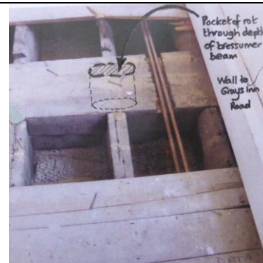
Fig 6 Floor structure in Office East side of First Floor & pocket of rot in bressumer beam
