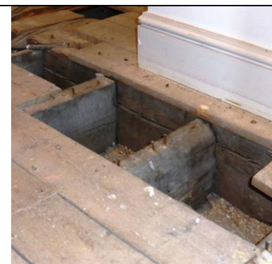
Fig 8 East/West bressumer beam below Hall spanning to Grays Inn Square external wall
