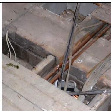
Fig 7 Existing split bressumer beam/ junction to centre beam below the Hall flooring
