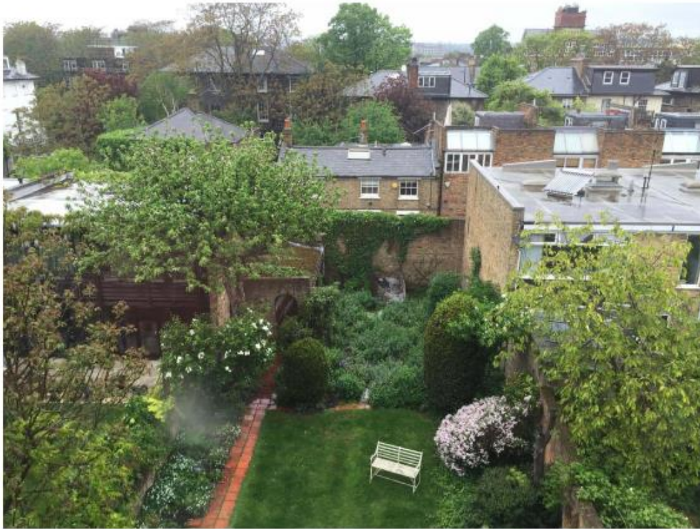
③ View of the site showing the existing brick wall and the derelict garage to be demolished.
