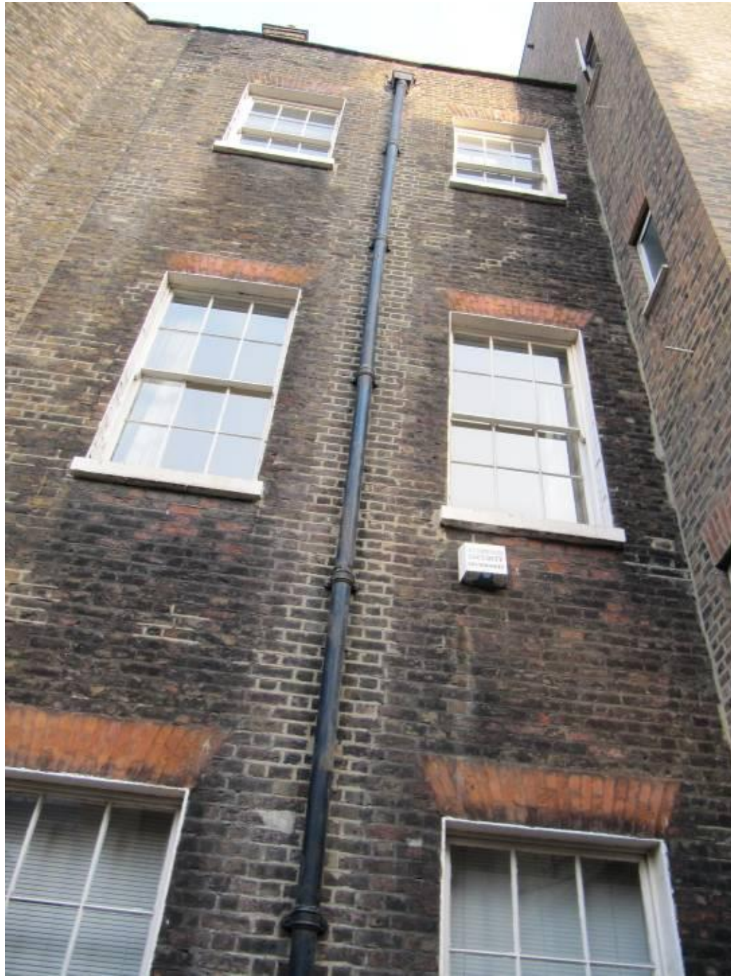
Existing Single Glazed Sash Windows to Rear façade (First, Second and Third Floors) Photo taken from Rear Lightwell
