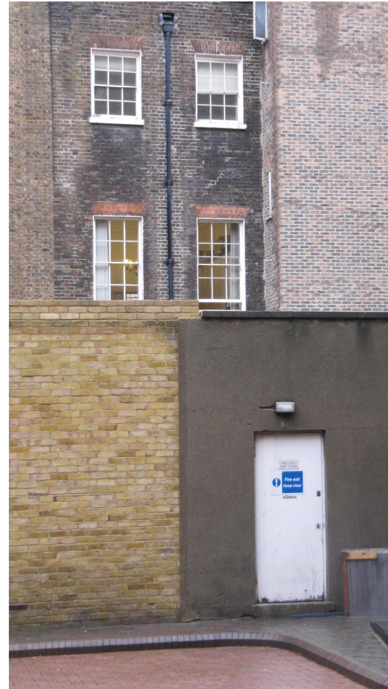
Existing Single Glazed Sash Windows to Rear façade (Second and Third Floors) Photo taken from Rear Car Park behind the application site
