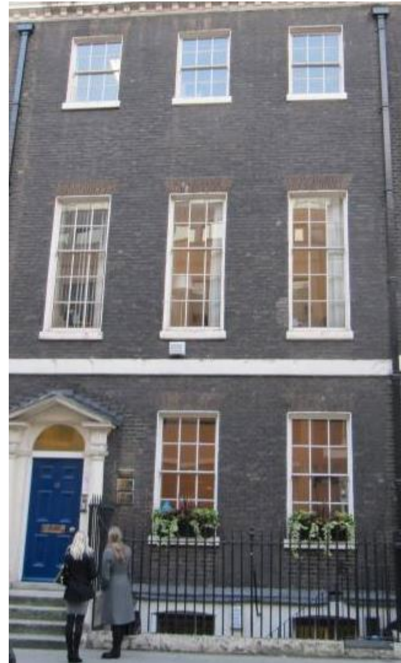
Existing Single Glazed Sash Windows to Front façade (Ground, First and Second Floors) Photo taken from Southampton Place
