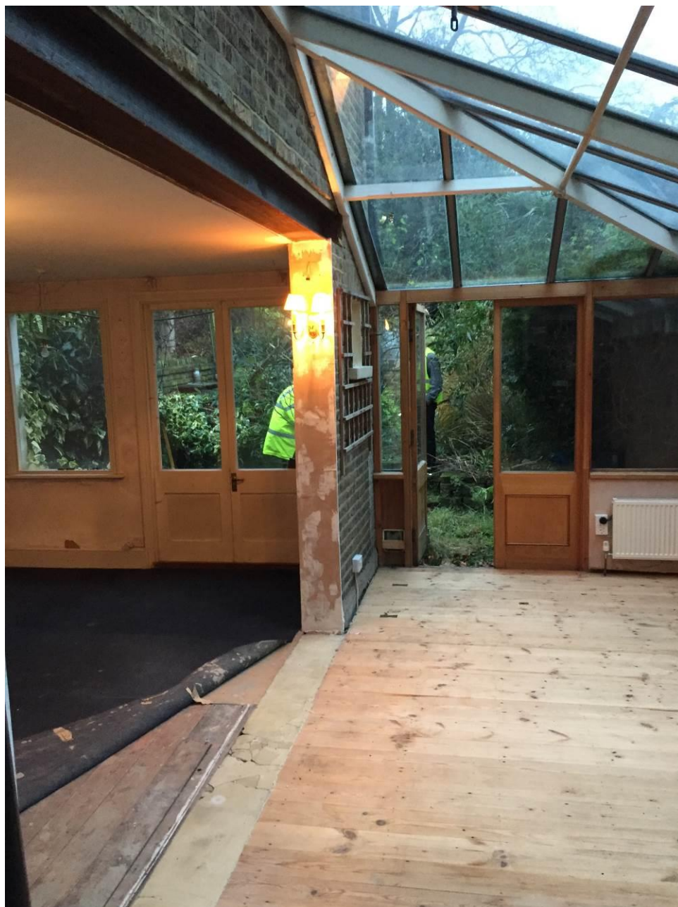
Photograph 3. Detailing the internal structure of the building looking towards the rear garden area
