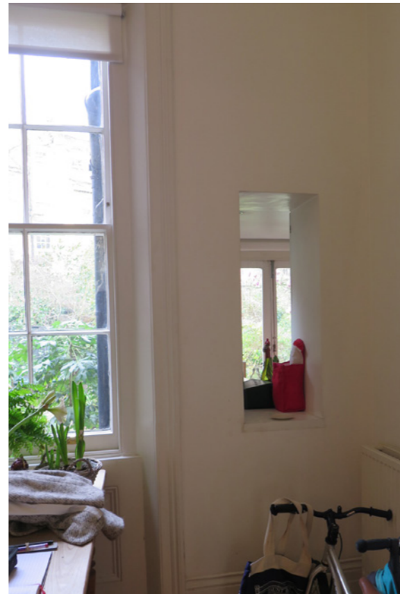
Detail of window to be lowered (architrave to be retained) & hatch to be infilled.
